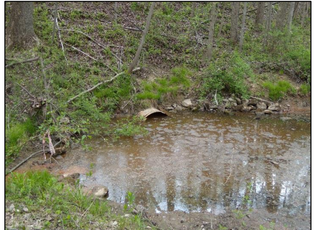
Photo 15. Outfall 2d, with silted channel backwatering the pipe.
