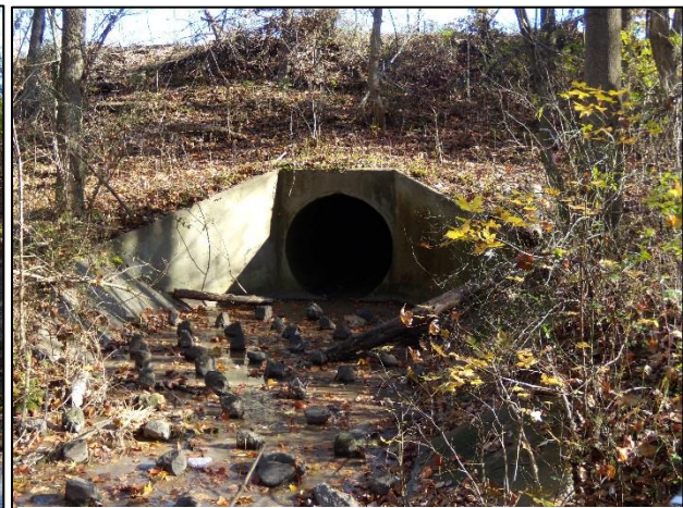
Photo 11. Outfall 2 draining to top of Central Dorsey Run
