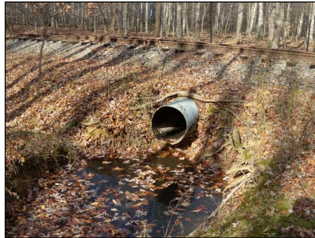
Photo 9: Stand 4 ephemeral channel entering the hub through a culvert under the railroad tracks.
