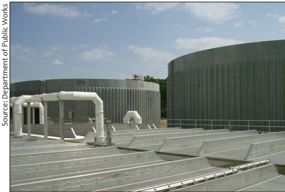
Wastewater pretreatment, such as at this industrial facility on US 1, can help reduce flow and nutrient concentration in flow sent to wastewater treatment plants.
