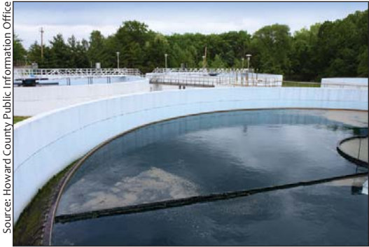
The Little Patuxent Water Reclamation Plant treats wastewater for about 70% of the County served by public sewer.
