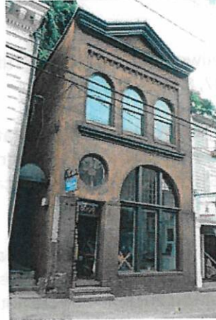
Figure 30 - Damage from 2016 flood
