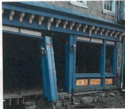
Figure 33 - Damage from 2016 flood
