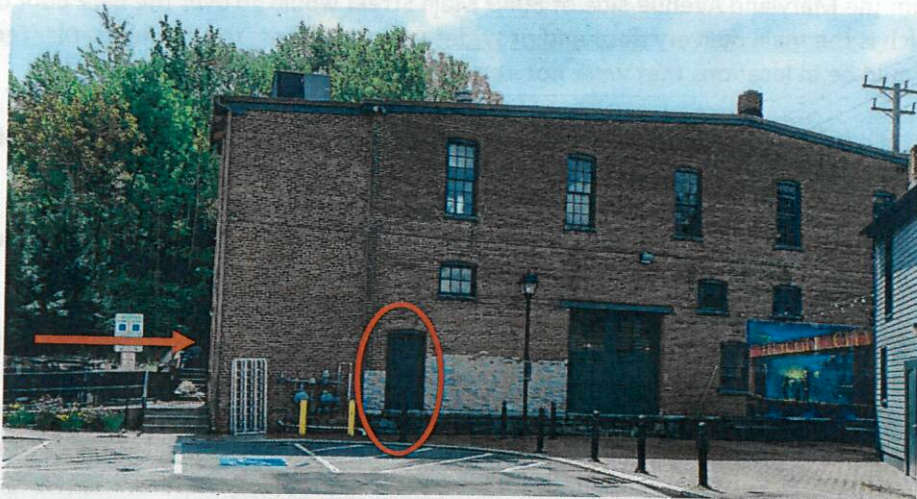
Figure 15 - Red arrow points to rear metal door and red circle shows side door. Please note – the colored brick around the red circle is only chalk.
