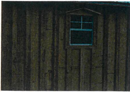
Figure 8 - Proposed board and batten siding, to be painted white, for all outbuildings.
