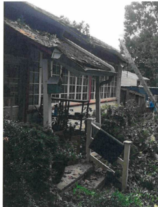
Figure 11 - Damage to building
