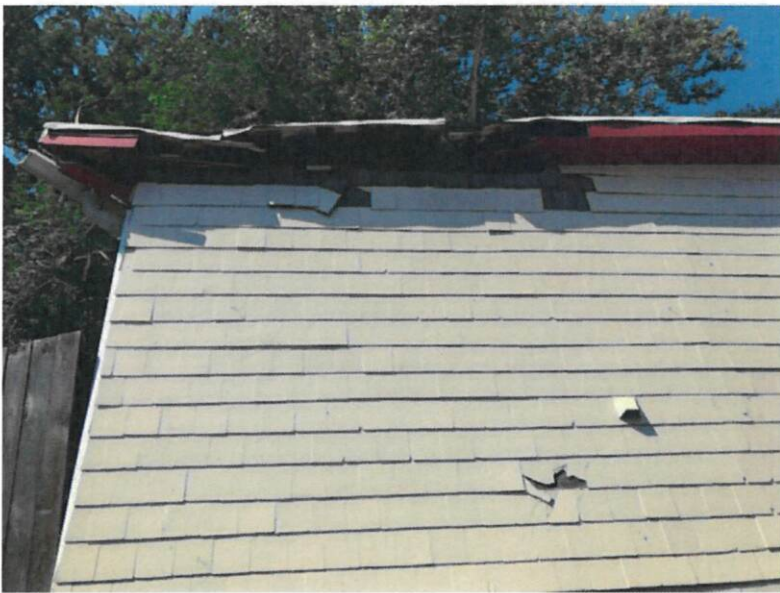
Figure 10 - Damage to asbestos shingles
