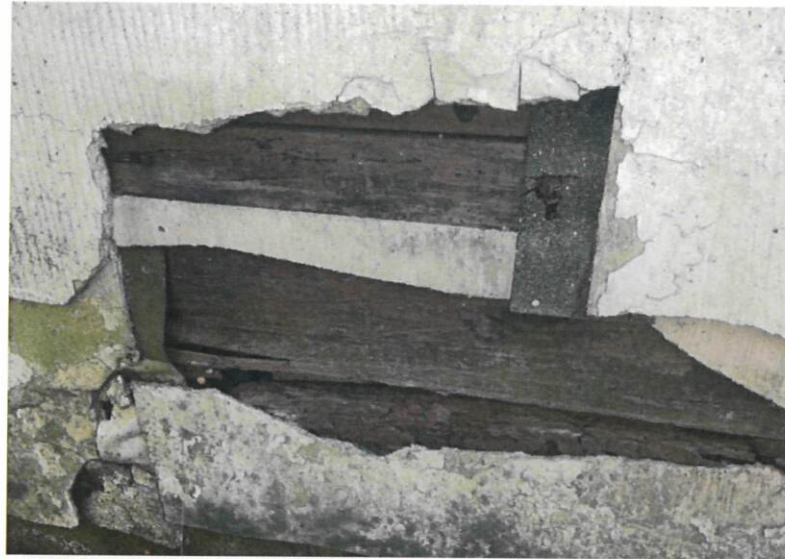
Figure 5 - Wood visible under asbestos.
