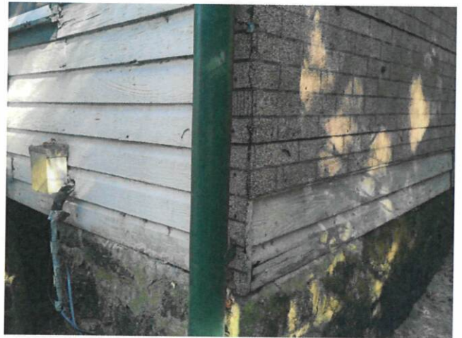
Figure 7 - Existing German lap siding, brick mold shingle and German lap siding under brick mold shingle.
