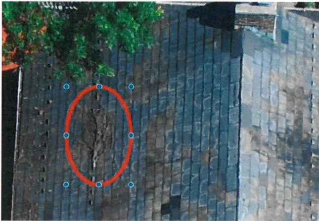
Figure 11 - Aerial view of roof damage.
