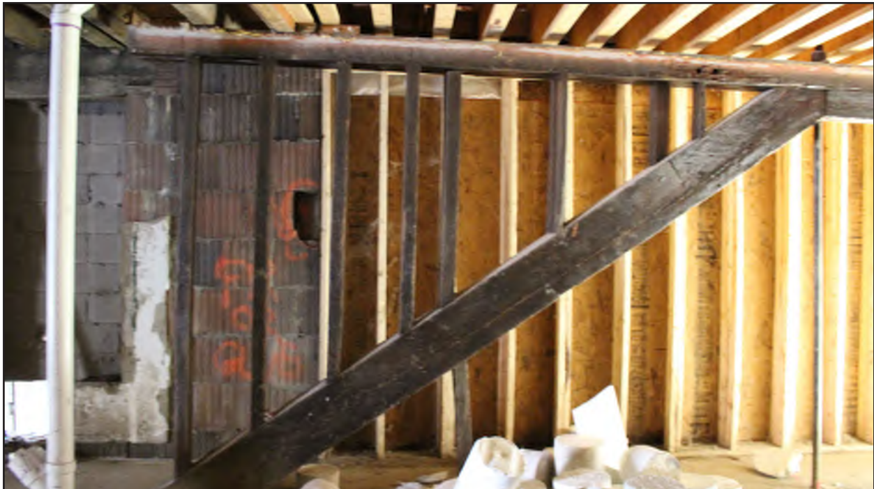
Figure 11: One of the timber supports that span the interior of the building
