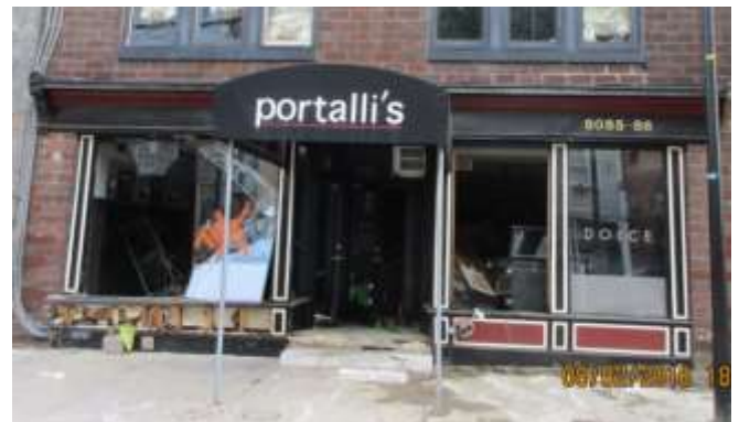
Figure 40- Front facade after flood 2016
