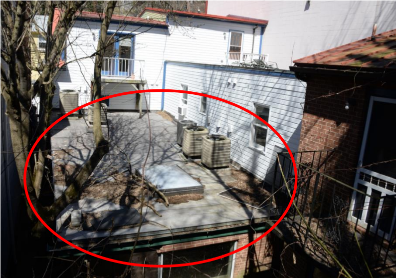
Figure 56 - Roof to be replaced
