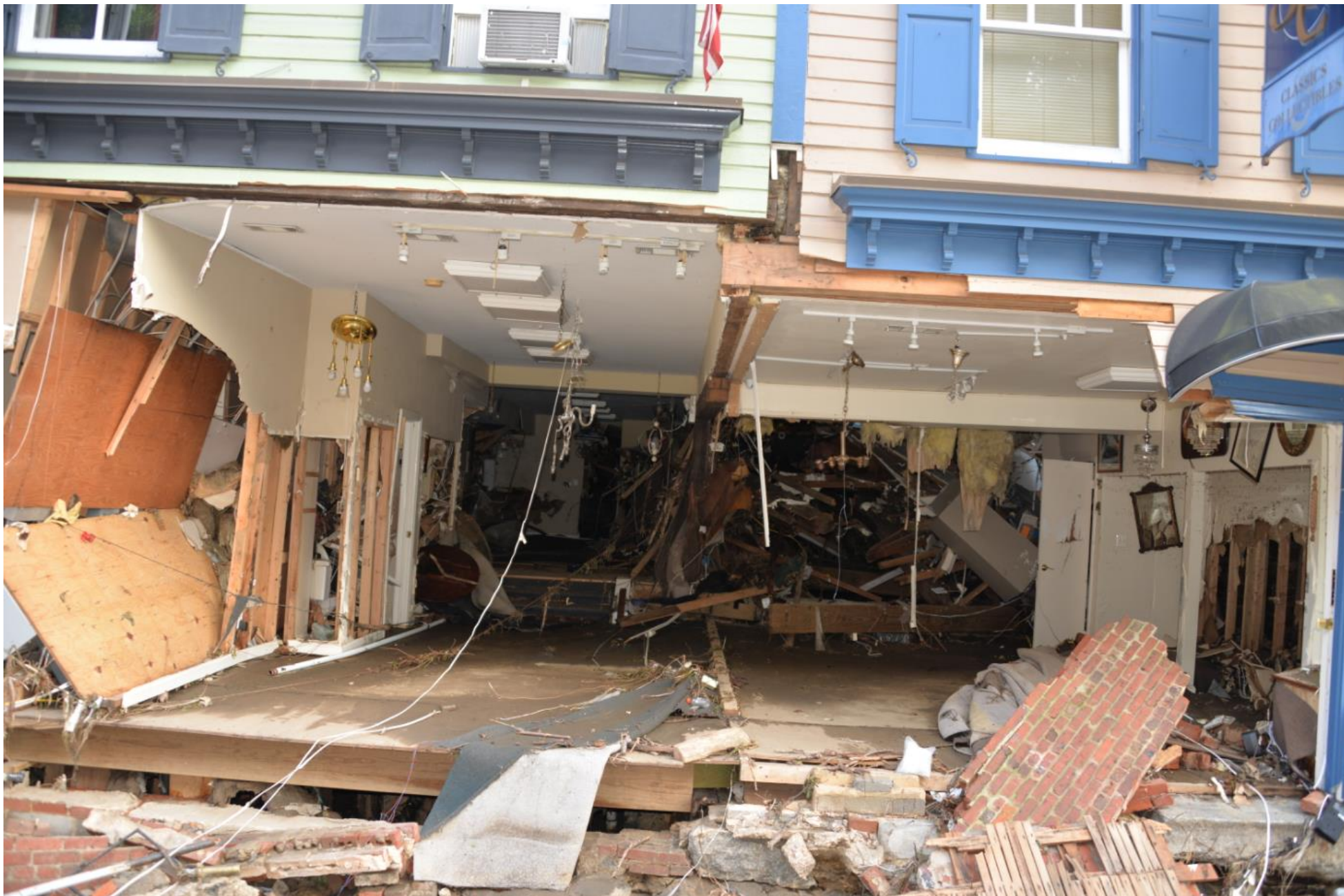
8109-8113 Main Street Johnson's Building 2016 Flood Damage
