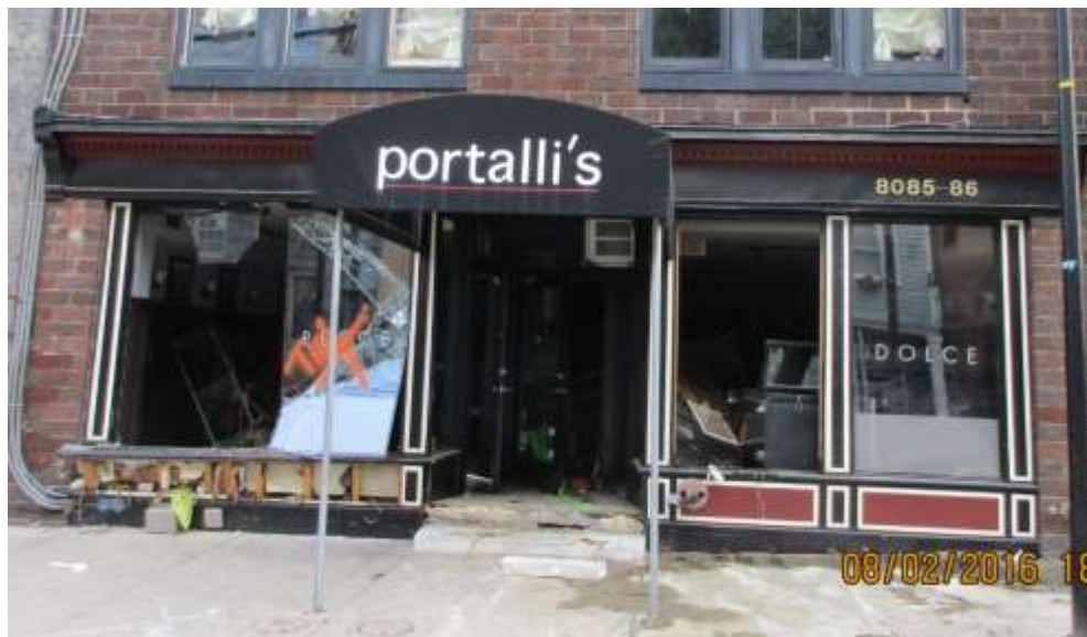
Figure 34 - Front facade after flood
