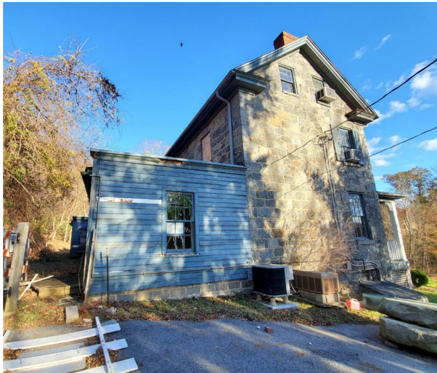
Figure 13 - Existing west view of the structure as seen from the upper part of the driveway/parking lot.
