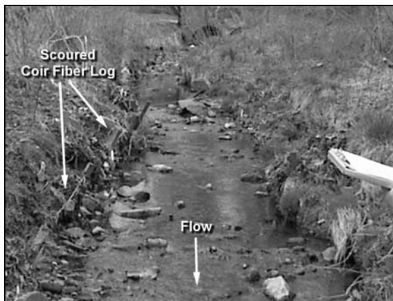
Figure 3: Coir fiber log has decayed without vegetative stabilization
