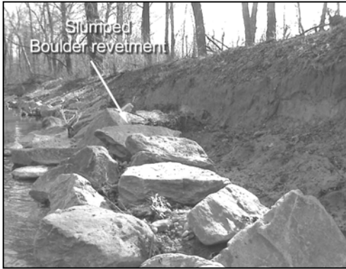
Figure 4: Boulder revetment failure due to toe scour
