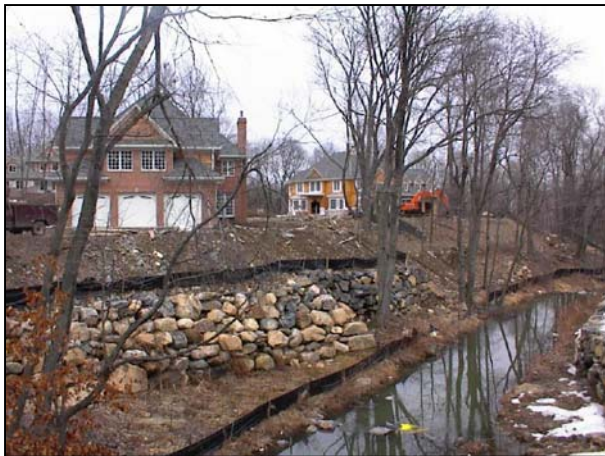
Figure 1: A New Subdivision Encroaching on the Stream Buffer
