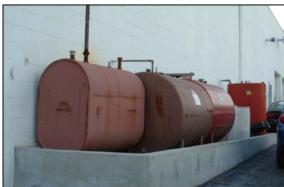
Figure 2: Secondary Containment of Storage Drums Behind a Car Repair Shop
