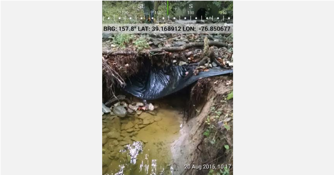
Downstream of the outfall pipe, in background of photo where erosion starts.
