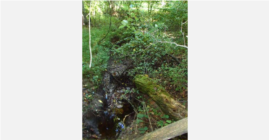
The eroded segment of the outfall looking downstream from the box elder.
