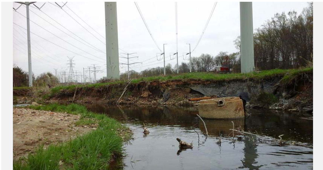
Facing downstream, existing channel where a deep pool has formed and recent bank failure has exposed pipes and geotextile fabric.
