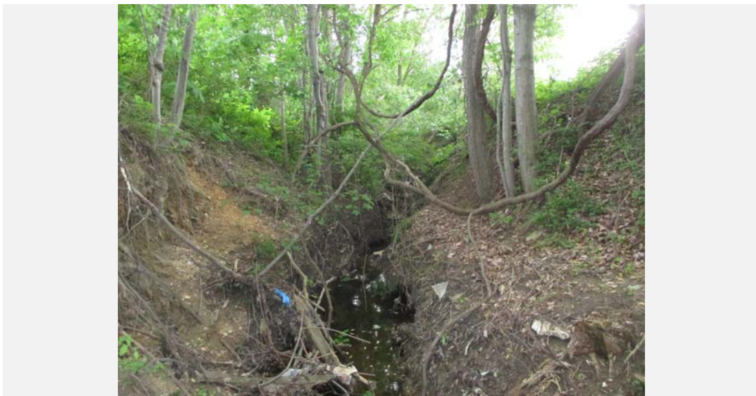
Erosion occurring along both banks of the incised tributary channel. Photo was taken looking upstream.
