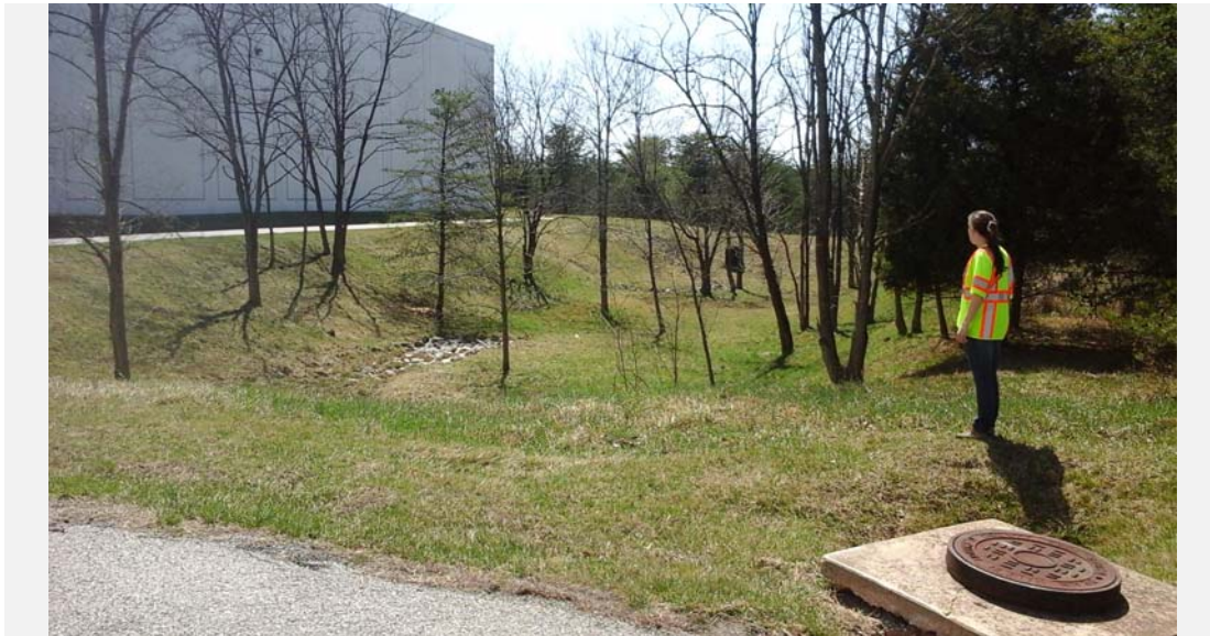
Looking south toward the facility from the asphalt access path. Failing manhole at bottom right of photo.
