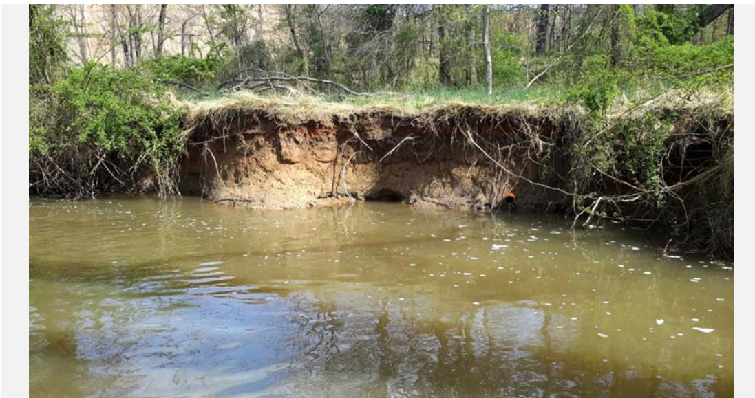
Facing the left bank, an eroded bank height greater than 5 ft. with no protective vegetative cover.
