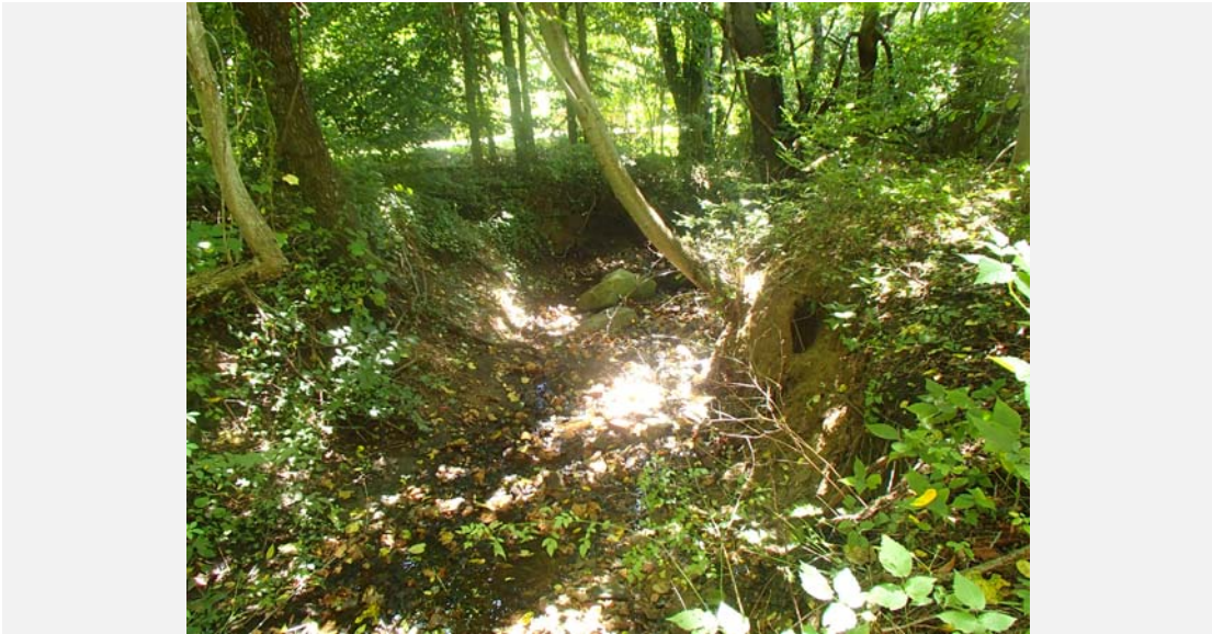
Eroded area downstream of outfall pipe.
