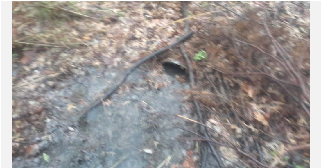
Facing upstream towards second outfall pipe with sediment deposition.
