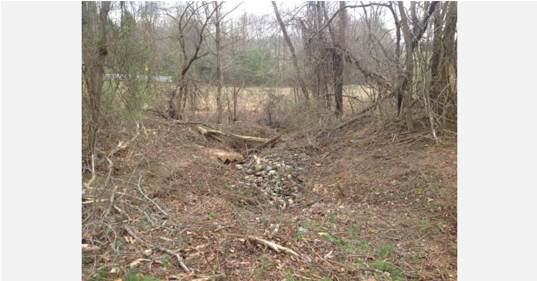
Downstream view from outfall showing eroded unstable channel.
