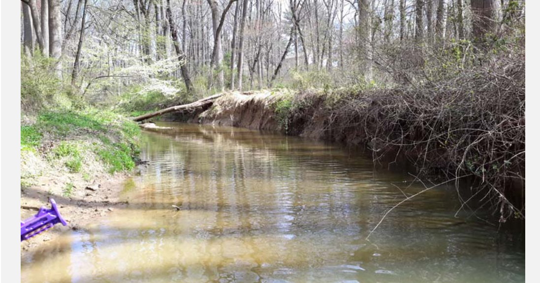
Facing upstream, evident bank erosion on the left bank (looking downstream).
