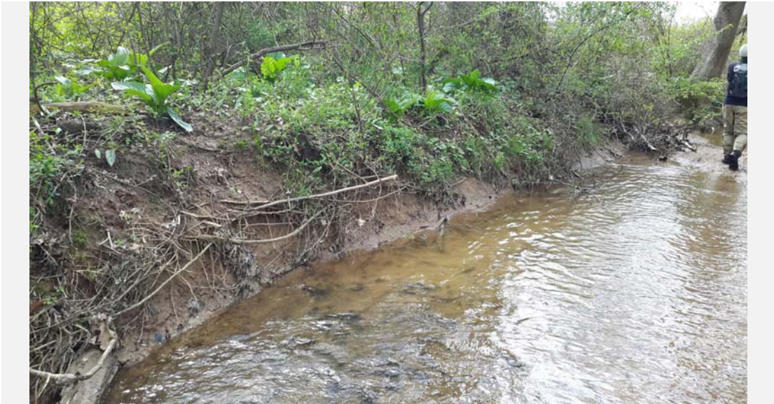
Facing upstream at the right bank showing average bank erosion for the site.
