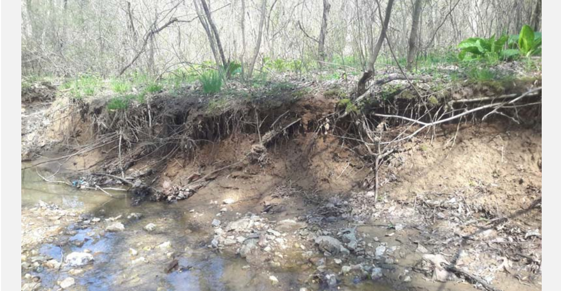
Erosion on right bank with vertical bank angle and poor root depth.
