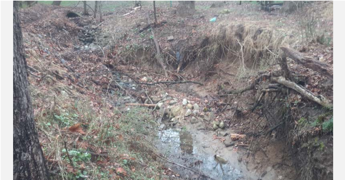
Facing upstream towards outfall, displaced riprap and eroded banks.
