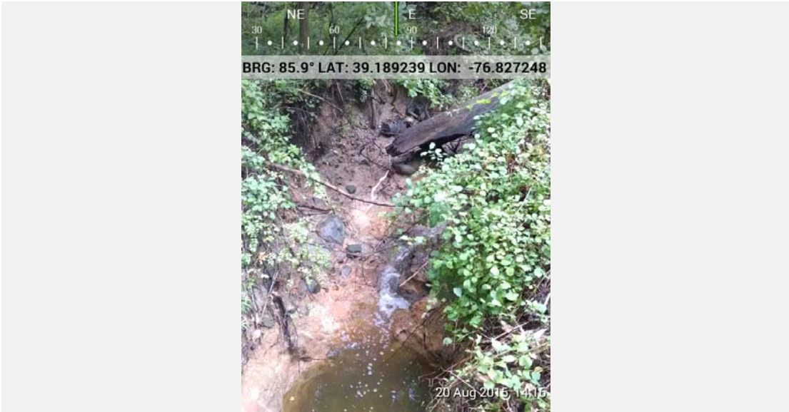
Area of erosion upstream of Patuxent Branch Trail.
