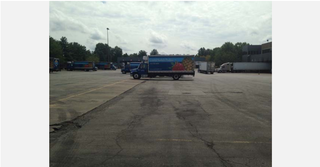
Standing on west end of north lot looking east. First of two at-grade inlets in foreground.
