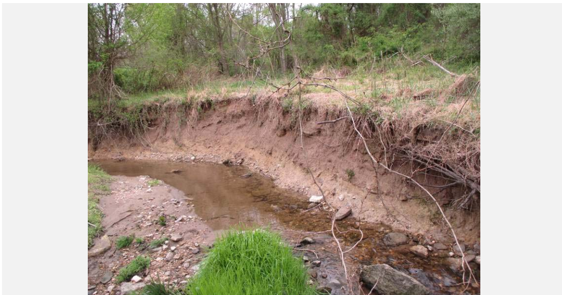
Erosion occurring along the left bank of the stream. Photo taken approximately 800 ft. upstream of Route 24. Bank height is approximately 5 ft.
