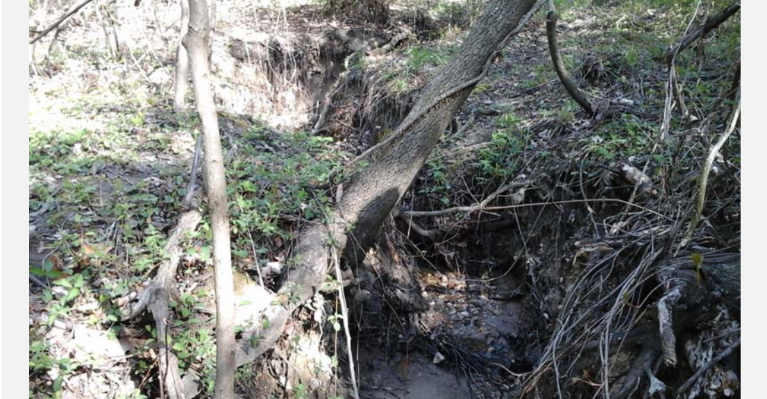
SR-52 facing upstream at erosion along the ephemeral reach.
