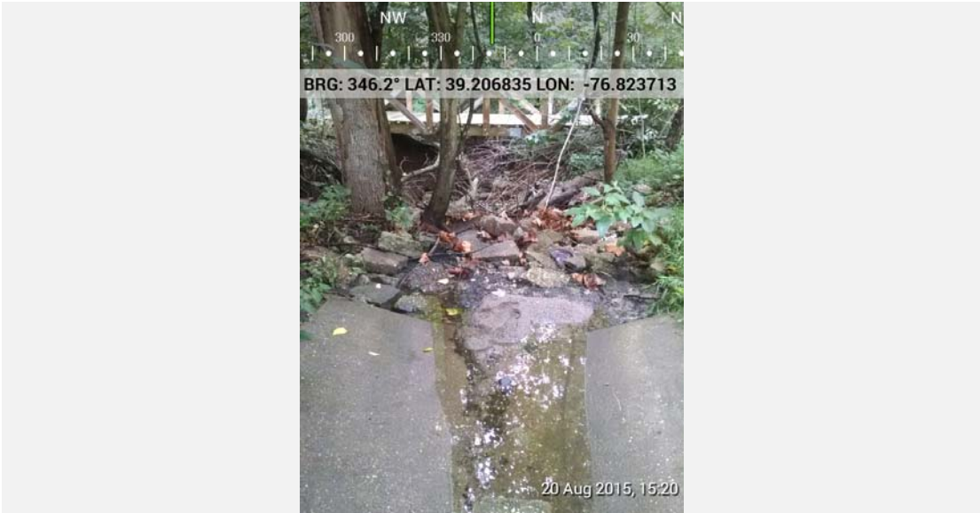
Standing on apron at outfall pipe looking downstream at drop and bridge for pedestrian trail.
