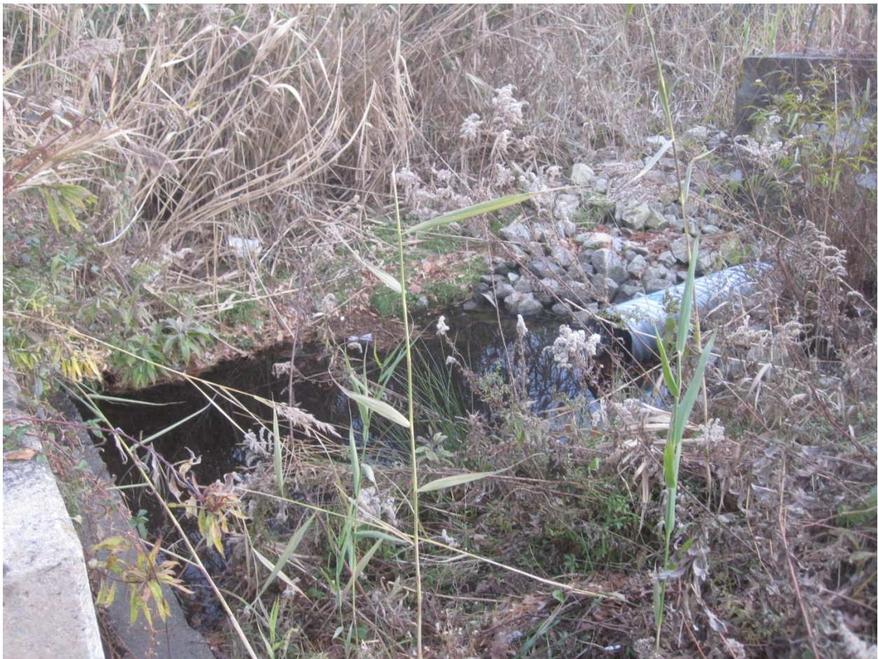
Figure 2. SWM pond at 6480 Dobbin Road, Dobbin Road Commercial Business Center, short circuiting dewatering structure, SLP-BC-D792
