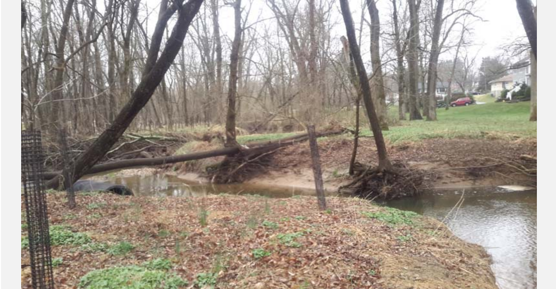
Eroding and undercut banks; fallen trees; poor quality riparian zone along right bank.
