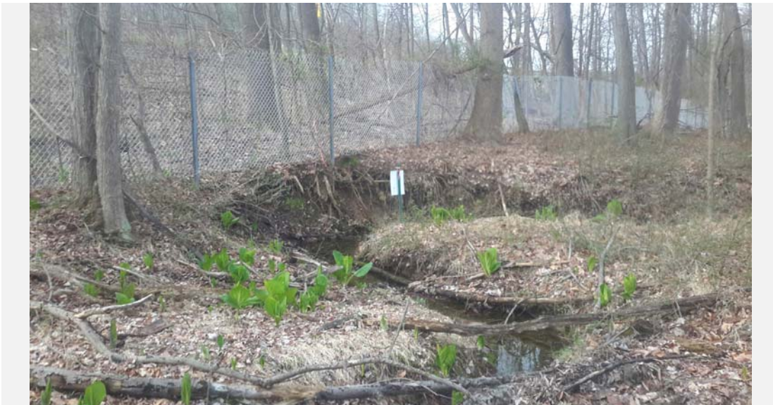
Facing downstream from outfall, bank erosion along outer meander bends.
