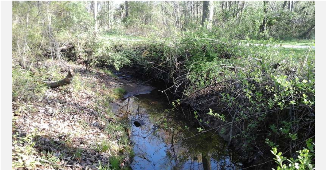
SR-52 facing upstream at bank erosion adjacent to the community trail.
