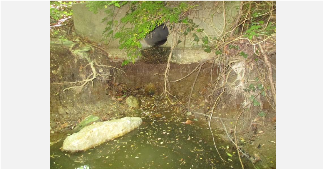
A 15 in. diameter concrete outfall headwall that is in need of replacement. The outfall currently sits 2.5 ft. above the bottom of the stream bed.
