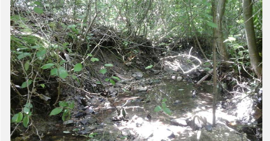
Erosion occurring along both stream banks. Photo was taken looking downstream and approximately 100 ft. downstream of Brush Run. Bank height is approximately 3.5 ft.
