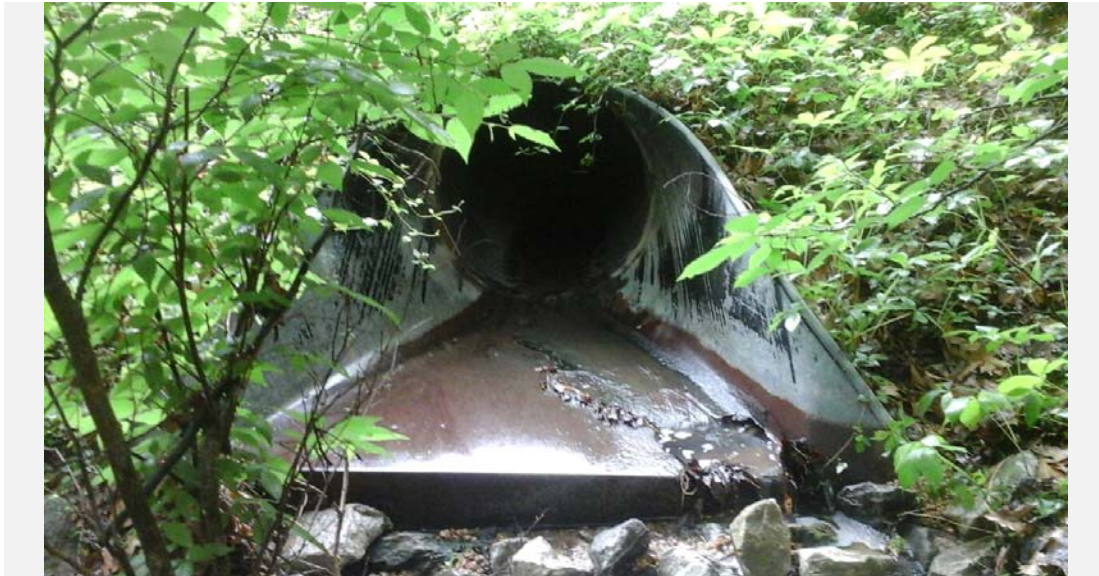
A 30 in. diameter corrugated metal outfall pipe with a rusted-out flared metal apron. The outfall drains a dry pond.
