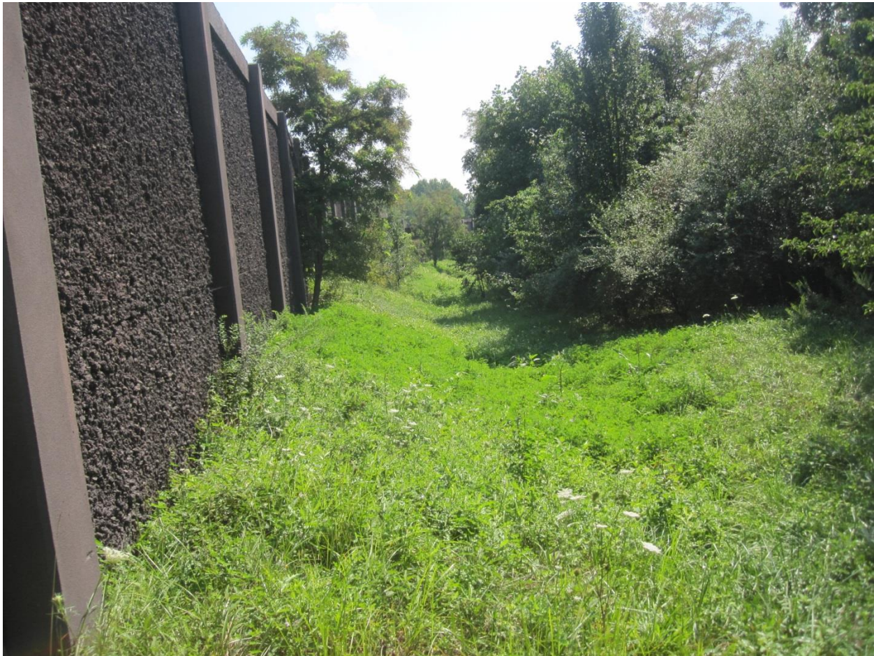
Figure 2. SWM pond at Crest Drive and Route 216, SMP-BC-D333
