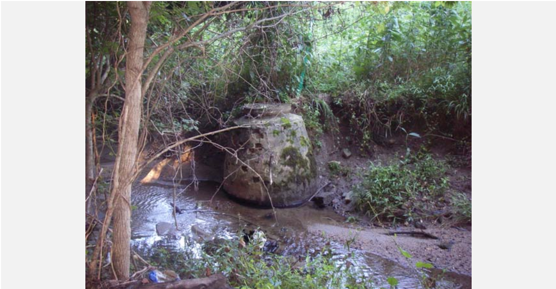
Close proximity to sewer line.
