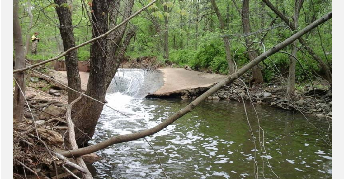
SR-59 facing upstream at failing dam structure.
