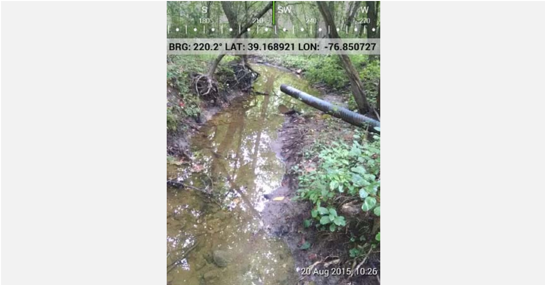
In the eroded area looking downstream at second outfall pipe.
