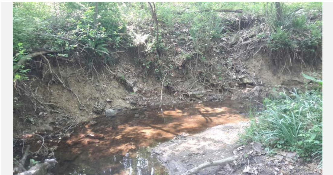
Reach 1, erosion on right bank.
