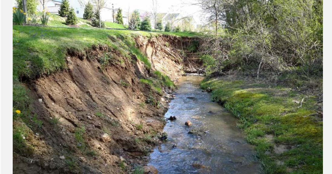
Facing upstream, a recent bank failure along the right bank (looking downstream), leaving the bank raw with little to no vegetative protection.
