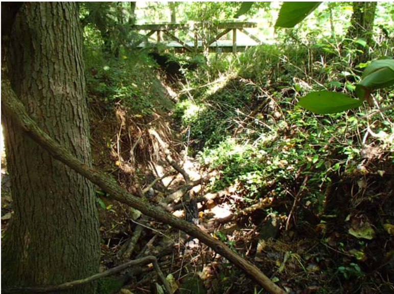
Standing downstream of pedestrian bridge looking at eroded area.
