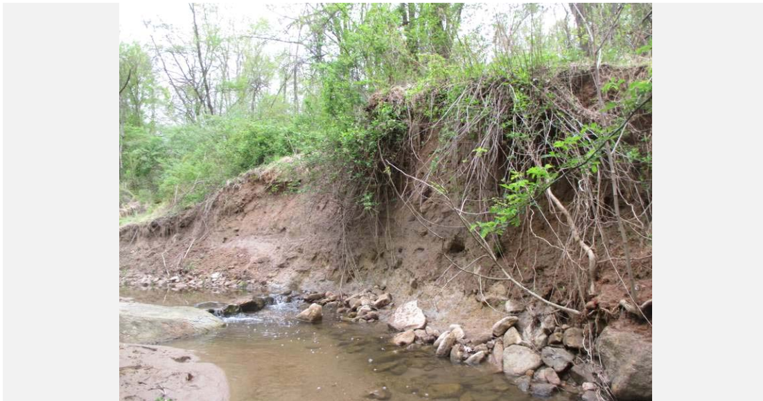
An approximately 7 ft. high sediment deposit located along the left bank. Sediment appears to have accumulated behind an old dam. Dam remnants can be found approximately 500 ft. upstream of Route 29.
