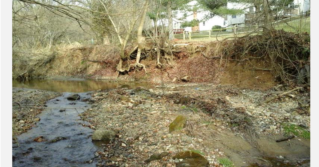
Erosion occurring along the left bank. Private residential yards with no trees are nearly abutting the stream in this section of the reach. Bank height is approximately 4.5 ft.
