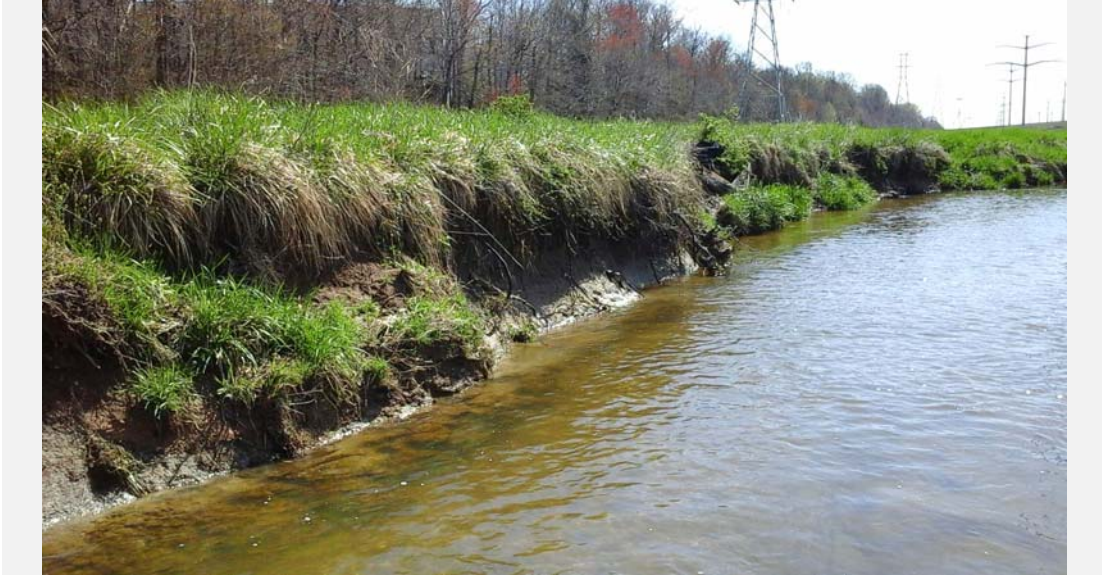
Looking downstream at recent bank failure along the left bank.
