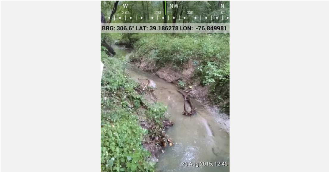
Standing on bank downstream of outfall pipe in eroded area.
