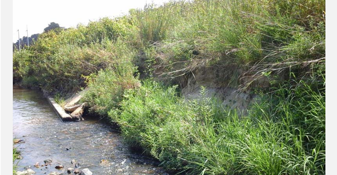
Facing downstream, an old concrete channel along the right bank that is causing bank erosion.
