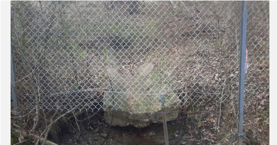
Facing upstream towards the outfall, severe erosion at the bottom of the concrete channel.
