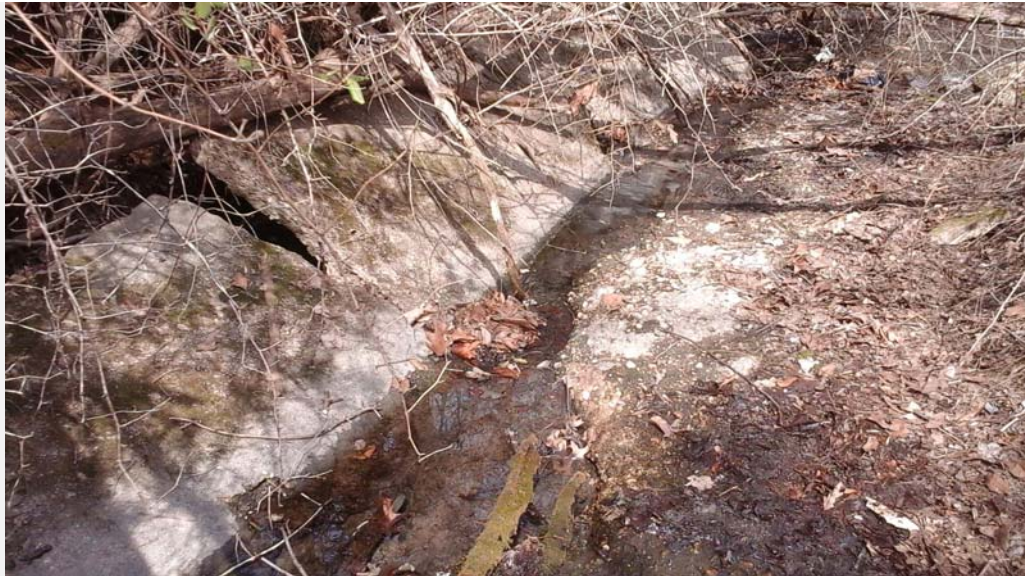
Failing concrete channel downstream of 36 in. outfall. Photo taken looking downstream.
