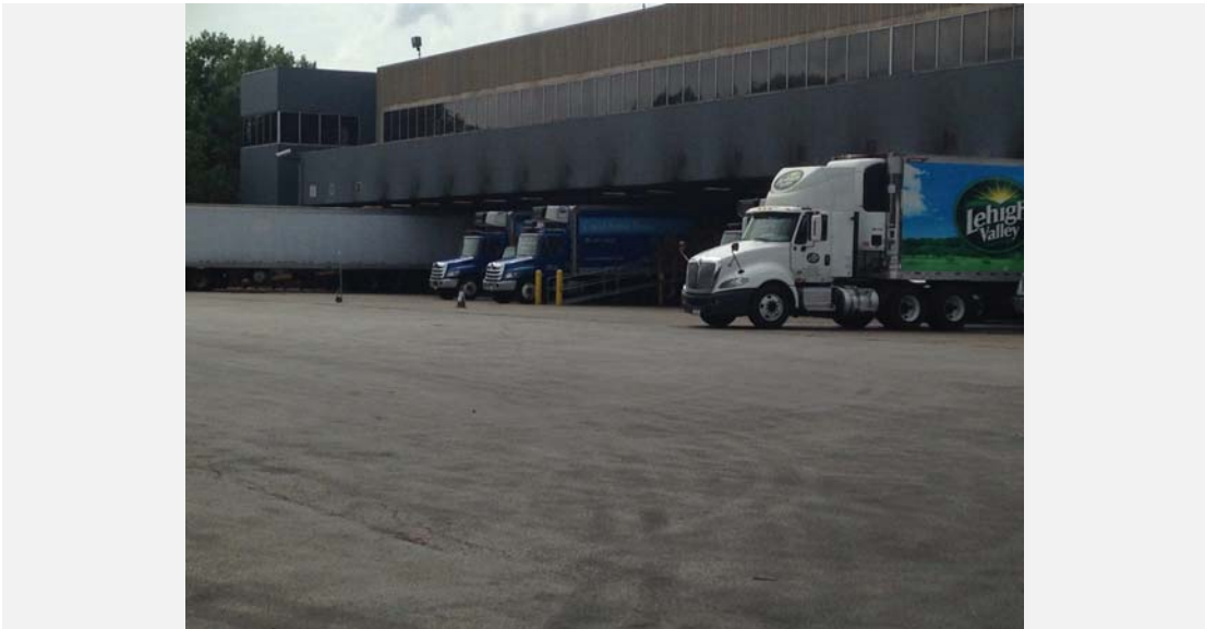
Independent stormwater system for docking bays evident by concrete sloping back to slotted drain along docking bays.
