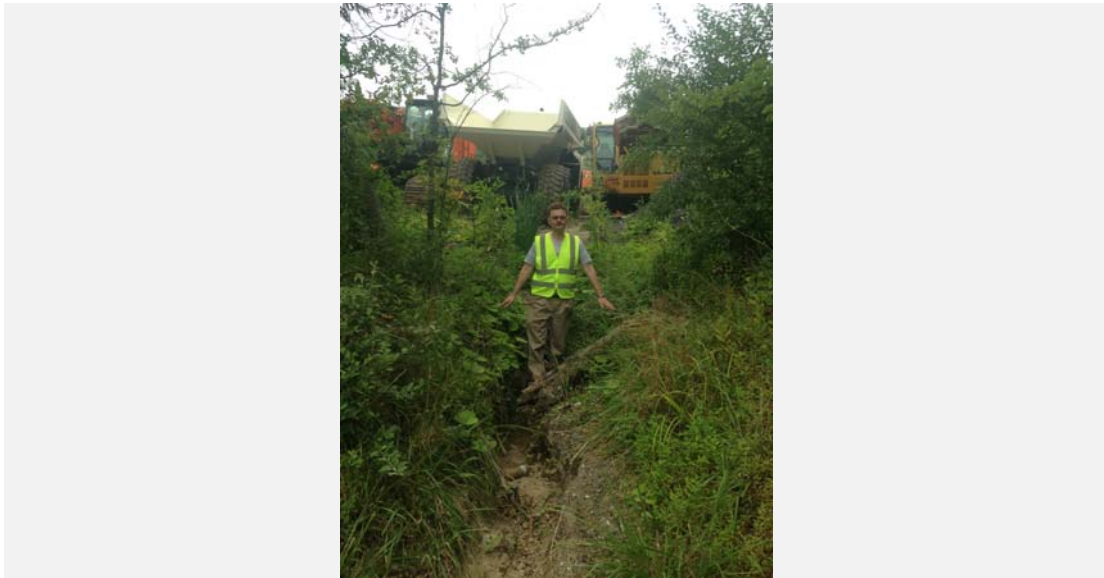
The erosion of the inflow swale.
