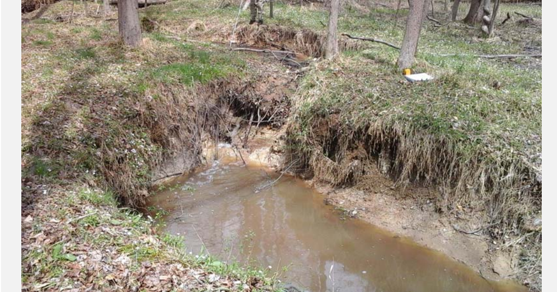
Facing upstream showing 4 ft. a headcut causing more extensive erosion downstream.
