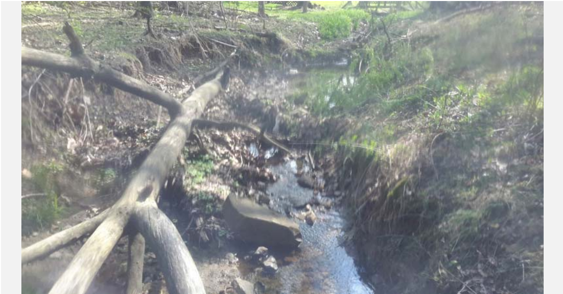
Facing upstream at headcut.
