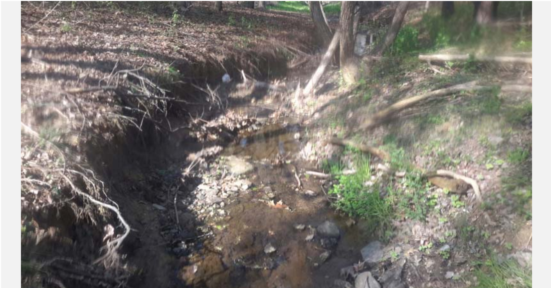
Facing downstream, erosion along outer bends.
