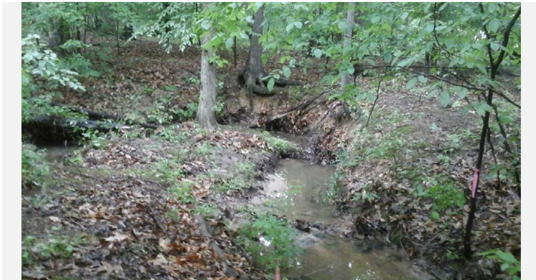
Minor to moderate erosion occurring around a meander bend in the outfall channel.
