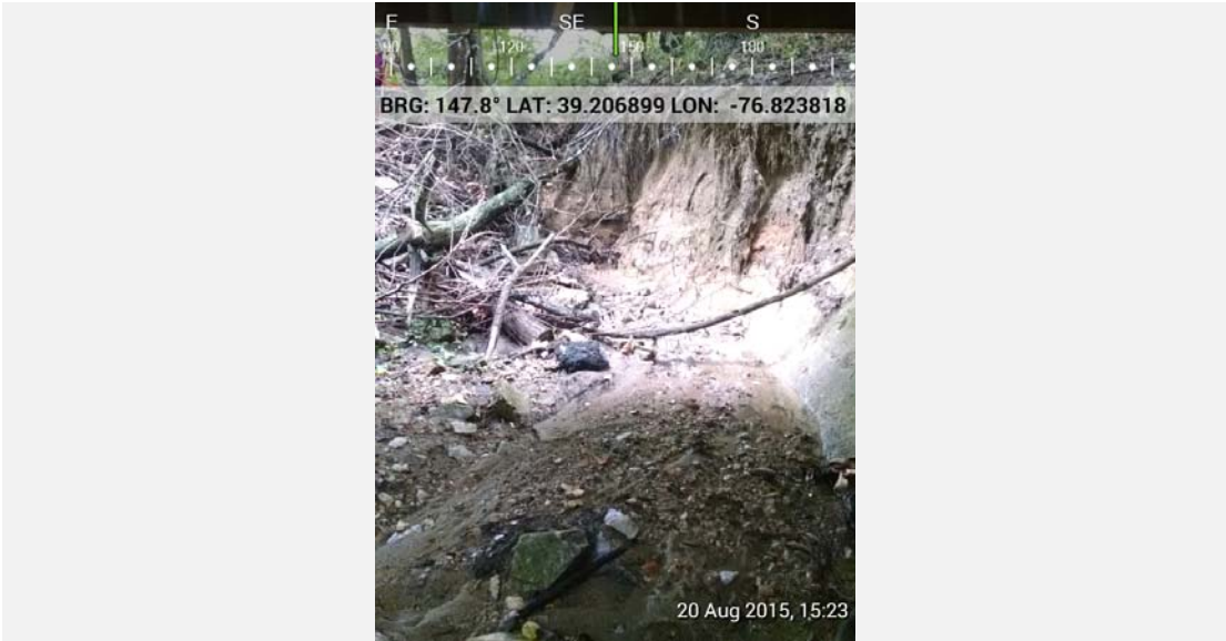
Standing under pedestrian bridge looking downstream at eroded bank.
