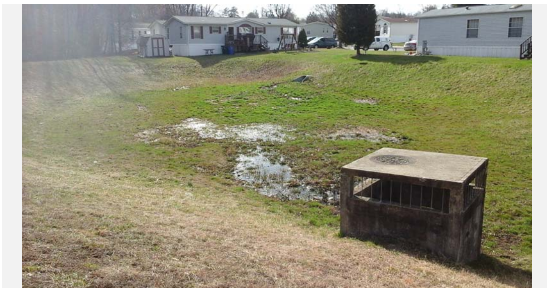
Looking west toward the riser structure and 24" CMP inflow from the pond embankment.
