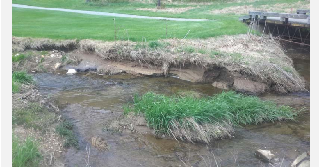
Left bank erosion with vertical banks, poor root depth and a silty material.
