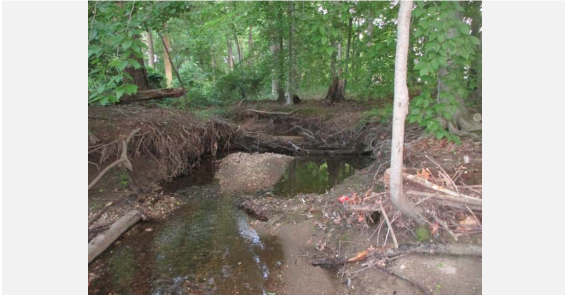
Erosion occurring along both banks of the mainstem. Photo was taken looking upstream.
