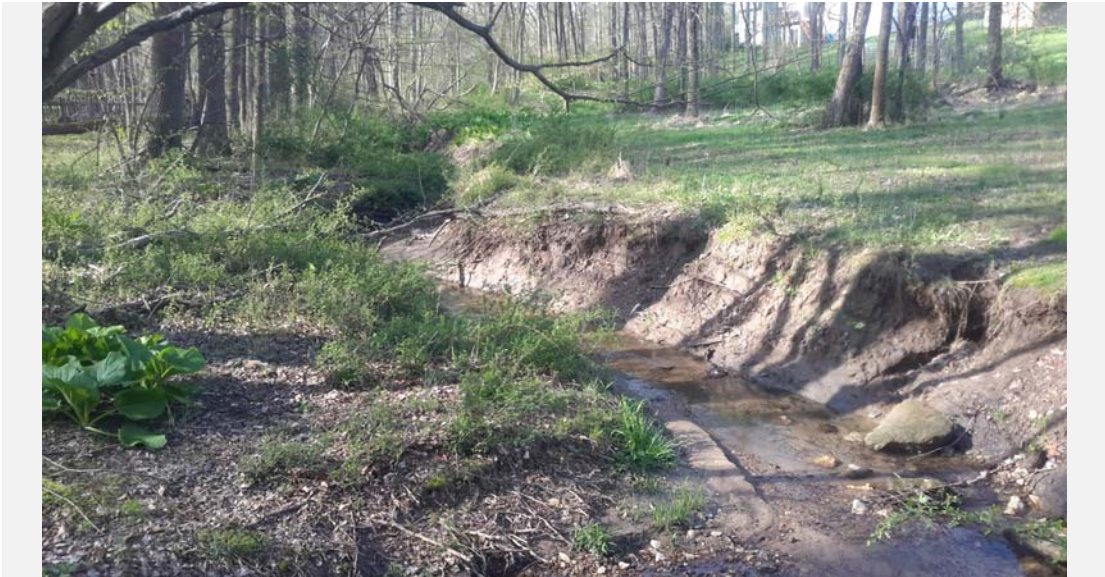
Right bank erosion with vertical bank angle, no surface protection and silty bank material.
