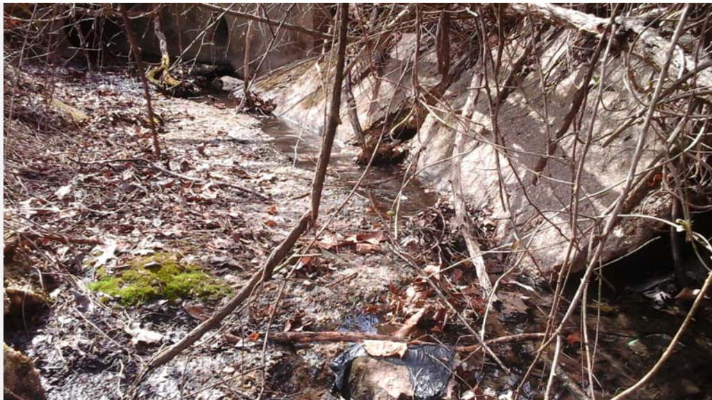
Failing concrete channel downstream of 36 in. outfall. Photo taken looking upstream shows that the stream is starting to cut around the left side of the concrete channel.
