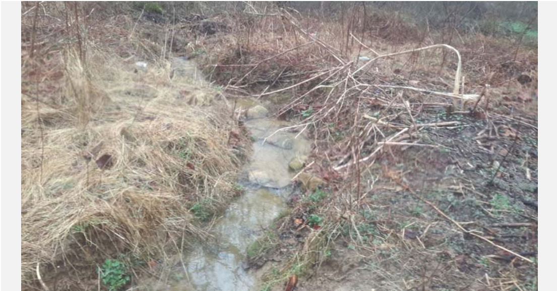
Facing downstream , above headcuts.
