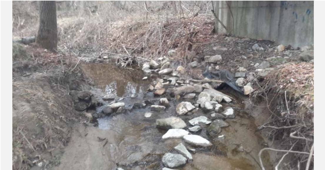
Failing riprap under footbridge.
