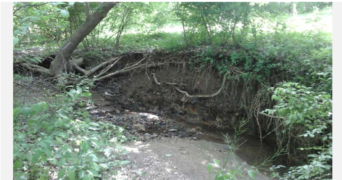
Erosion occurring along the left bank. Photo was taken close to the downstream extent of the proposed restoration reach. Bank height is approximately 4.5 ft.
