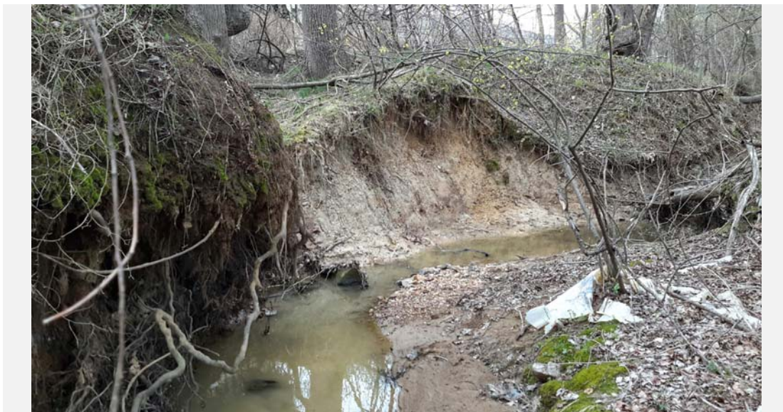
Facing upstream, variable bank heights with no bank protection and more fallen trees.
