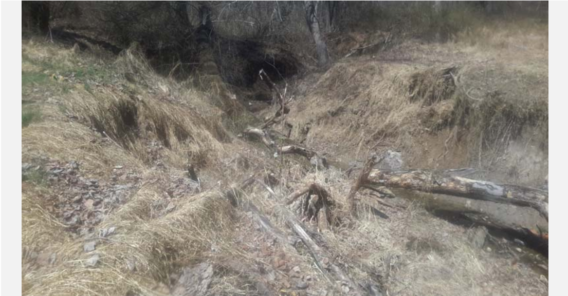
Vertical and eroding banks, severe erosion.
