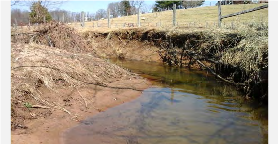
SR-5 facing upstream at moderate bank erosion that threatens existing infrastructure.
