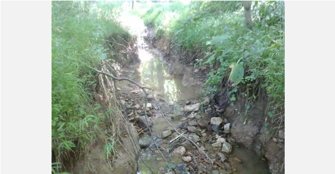
SR-60 facing downstream at moderate bank erosion.
