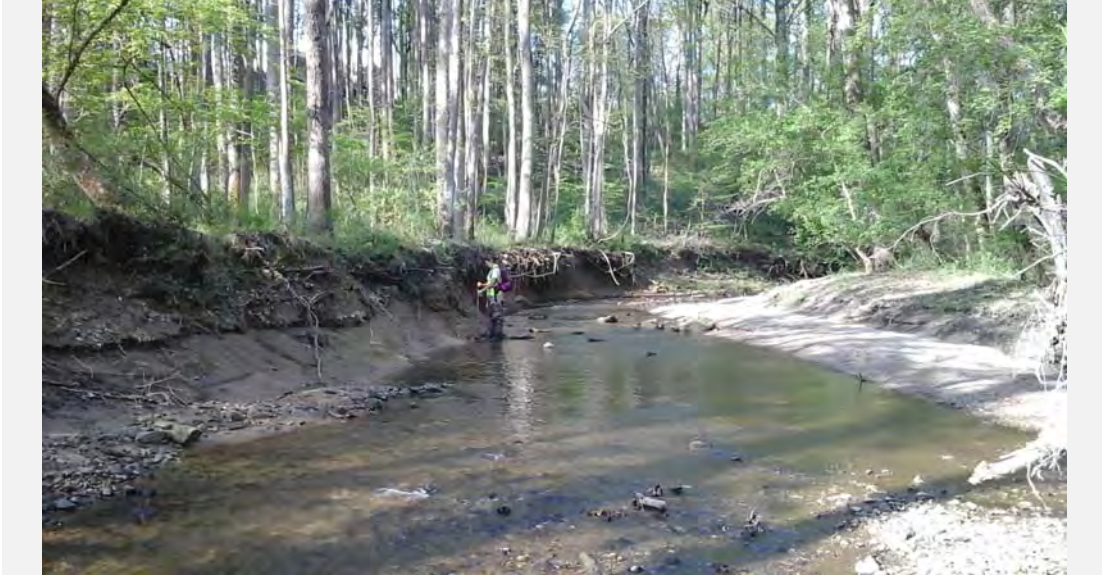
Facing upstream along the tributary (SMP-SR-F360A) showing little bank vegetative cover and protection along with large lateral bar formation.
