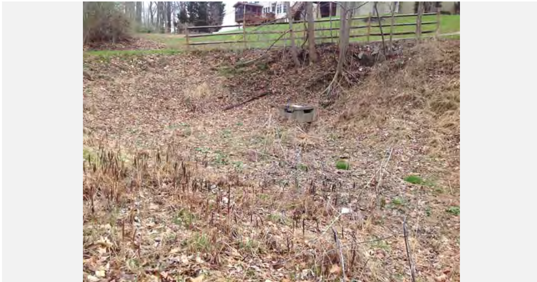
Infall to facility and eroded upstream slope.
