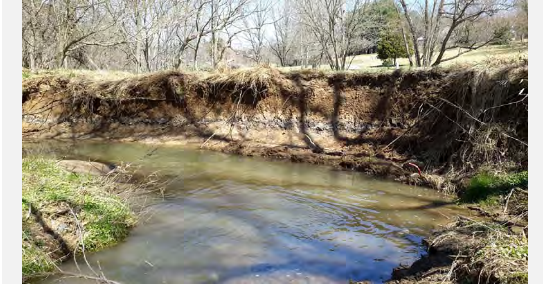
Facing downstream at a tight bend within the existing channel displaying poor bank protection, lack of vegetative protection and lack of riparian vegetation.
