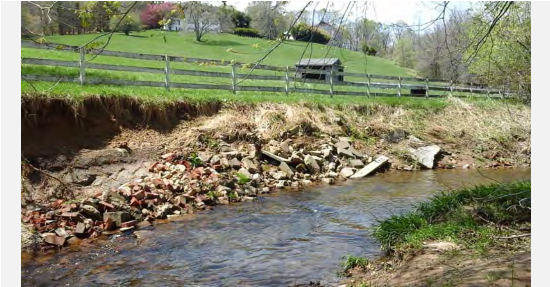
SR-12 facing upstream at severe bank erosion that is threatening existing infrastructure.
