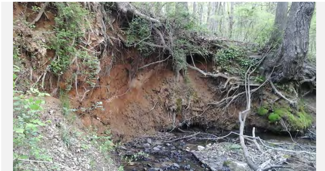
Looking downstream at a tight bend that has created an extremely high and raw left bank.
