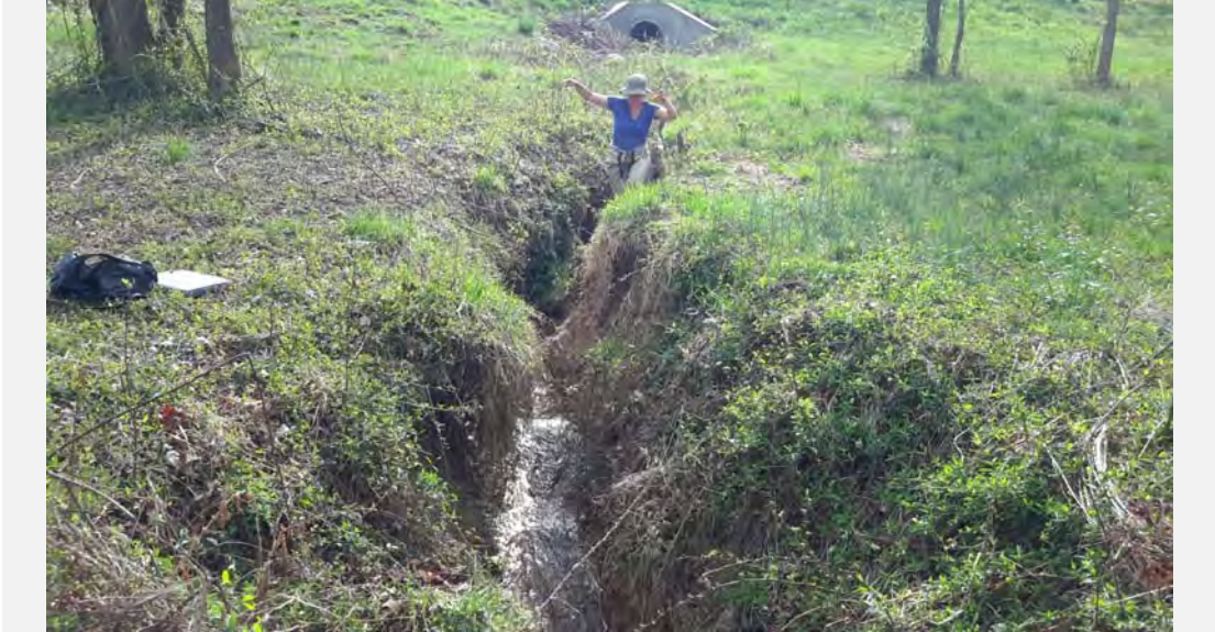
Facing upstream, the pond outlet and eroded discharge channel.
