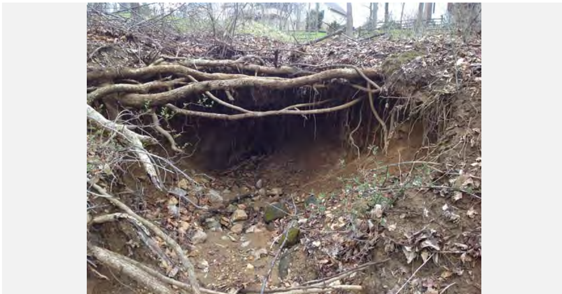
Looking upstream at outfall erosion just downstream of weir.
