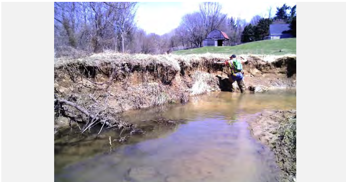
Facing upstream at another tight bend within the existing channel displaying poor bank protection, lack of vegetative protection and lack of riparian vegetation.
