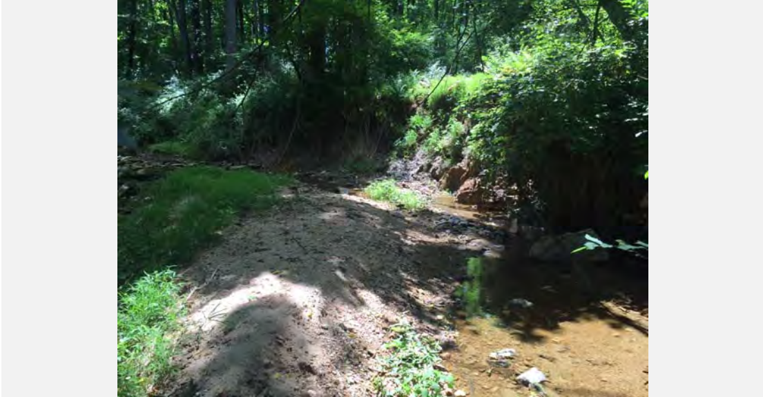
SR-60 facing upstream at severe bank erosion.
