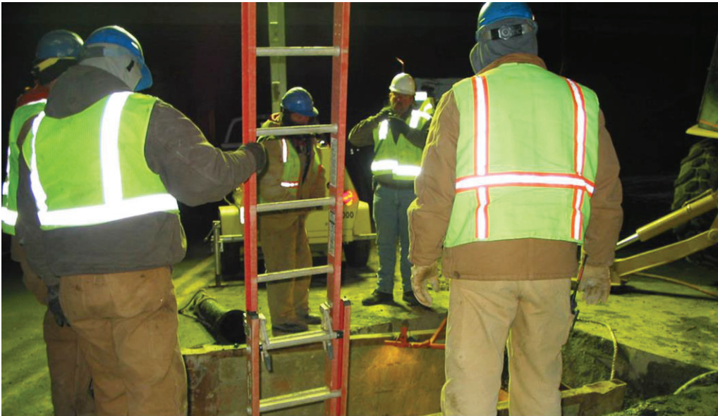
Bureau of Utilities System Maintenance Division maintains Howard County's public water and sewer system ensuring high quality water service and fire protection.
