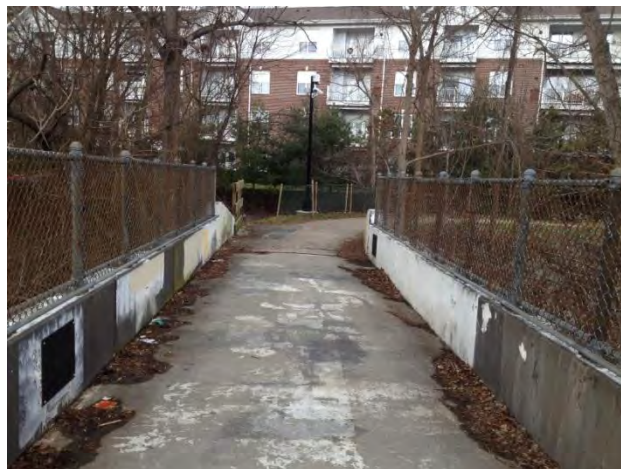
Photo 9: West Side Trail From West End of Pedestrian/Bicycle Bridge at Columbia Town Center Apartments (Facing West)
