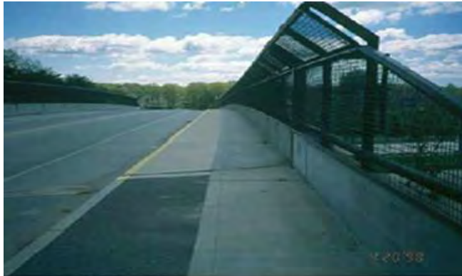
Photo 14: Typical SHA Vehicular Bridge Sample Condition with Chamfered Fence to Deter Thrown Objects
