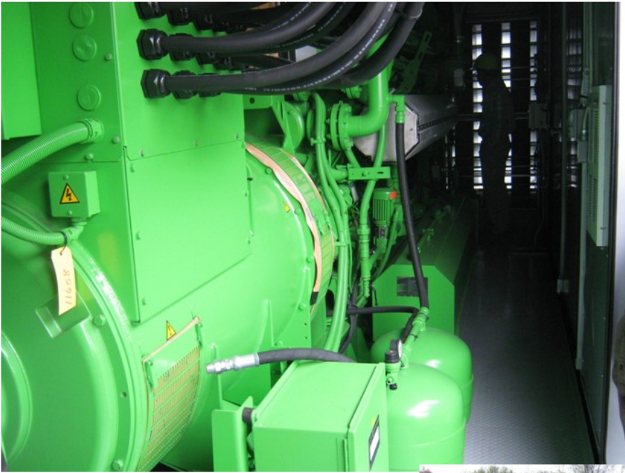
The gen-set, a Jenbacher J320, is housed inside of sound attenuated enclosure.
