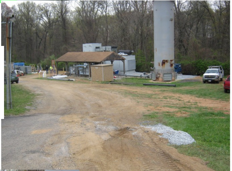
View of gen-set positioned behind existing blower station with air intake, radiator and exhaust silencer installed on top from left to right.
