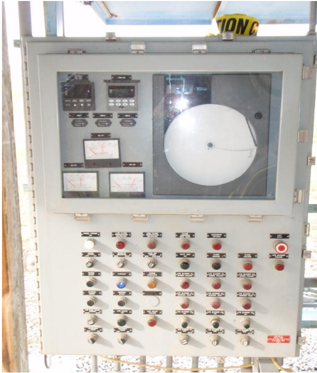
Existing Flare controls and shutoffs
