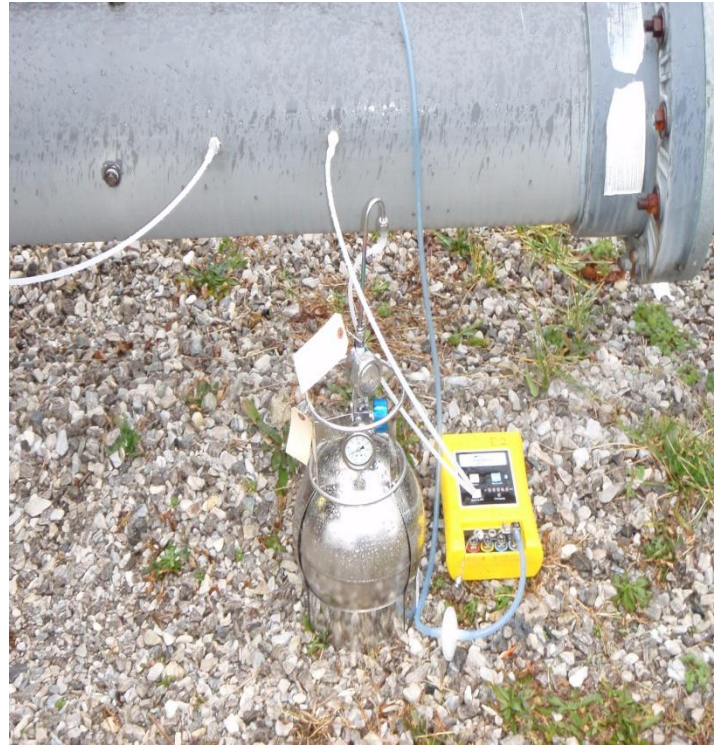
Influent testing for VOCs, mercury and methane
