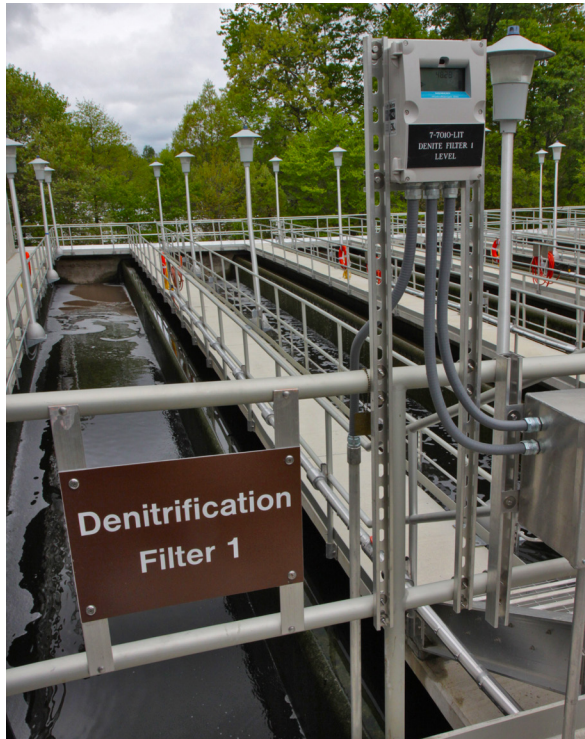
Capital investment in the County's wastewater treatment facilities is necessary for ensuring adequate capacity is available for projected population growth.
