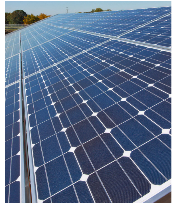
Solar panel demonstration projects such as this at the former New Cut Road landfill are located on a number of Howard County facilities. They save energy and promote sustainability.
