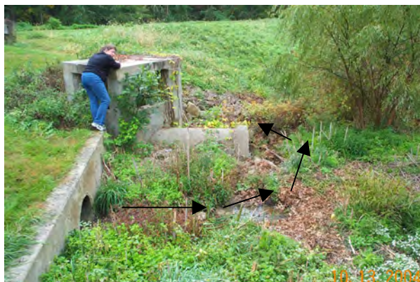
Figure 3.18 Short-circuiting at Beaverbrook stormwater pond.
