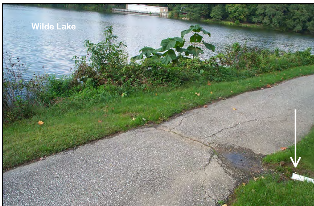
Figure 3.9 One of the more extreme downspout connections. Connection (see arrow) shown here has worn a small channel across the footpath that surrounds Wilde Lake.
