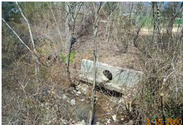
Figure 4.36 Eroding outfall from parking area/road.
