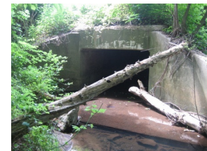
Point # 116 Location: -76.840603 39.278223 Description: Road crossing. Some debris at inlet.
