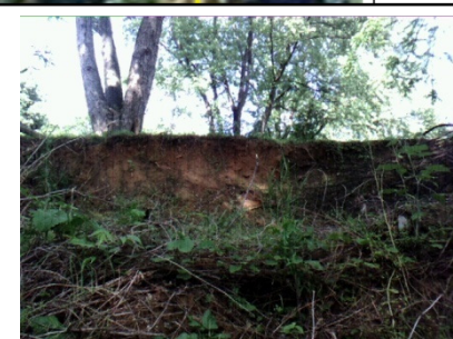
Point # 103 Location: -76.840812 39.279274 Description: Erosion site. Appears to have taken out a split rail fence.
