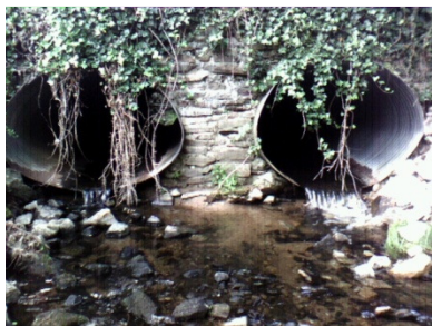
Point # 102 Location: -76.840877 39.279324 Description: Road crossing. Stacked stone headwall, ~8 feet above culvert inlet.
