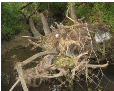
Point # 1062 Location: -76.820210 39.272175 Description: Debris blockage. Twin bole root wad in middle of channel.
