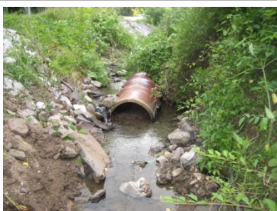
Point # 1078 Location: -76.822124 39.271855 Description: Old pipe in channel.
