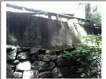
Point # 1015 Location: -76.800172 39.268942 Description: Failing cinderblock wall.
