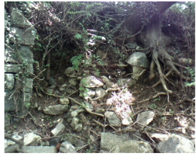
Point # 1014 Location: -76.799923 39.268748 Description: Failing bank, large amount of wall in stream.
