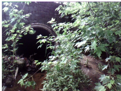
Point # 111 Location: -76.841346 39.280958 Description: Minor debris in right cell, excessive point bar formation with heavy vegetation immediately upstream of inlets of both cells. Stacked stone headwalls, ~8' above invert.
