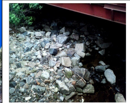
Point # 1003 Location: -76.795726 39.267545 Description: Debris blockage. Diverting flow directly into stone wall.
