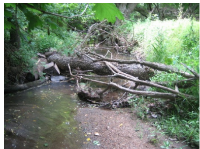
Point # 114 Location: -76.840765 39.278603 Description: Debris blockage. Creating some backwater.
