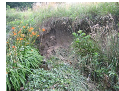
Point # 1060 Location: -76.819545 39.271980 Description: Erosion site. Lack of vegetation.
