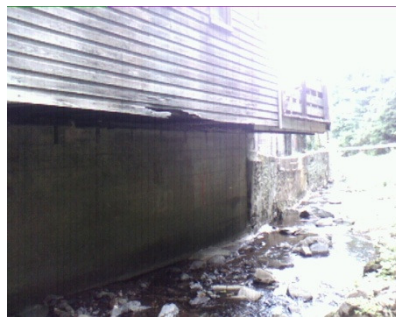
Point # 1033 Location: -76.808158 39.268503 Description: House overhanging stream.
