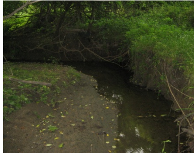
Point # 1074 Location: -76.821125 39.272177 Description: Erosion site. Outside meander.
