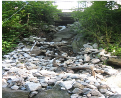
Point # 1007 Location: -76.798472 39.267226 Description: Failing riprap outfall to channel.
