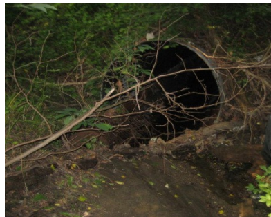
Point # 1073 Location: -76.820834 39.272047 Description: Debris blockage. Debris and sediment built up at inlet.
