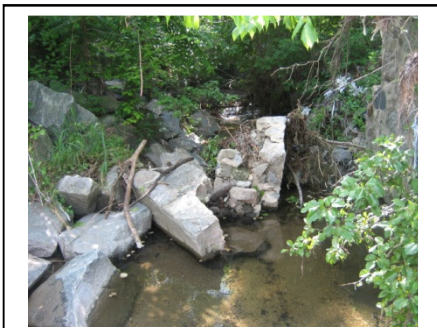
Point # 1039 Location: -76.810444 39.269121 Description: Debris blockage. Pieces of rock wall in middle of channel.
