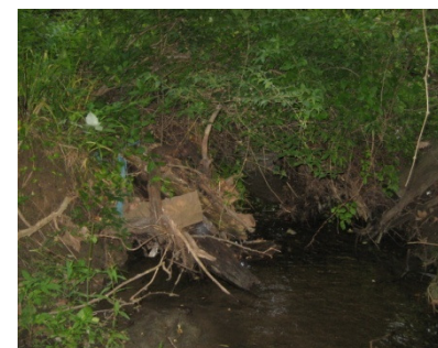
Point # 1075 Location -76.821333 39.272209 Description: Debris blockage. Various debris in channel.
