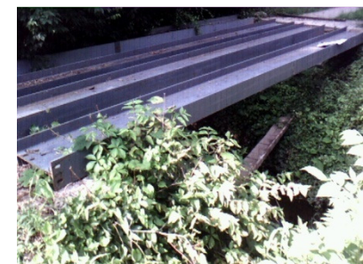
Point # 109 Location: -76.841102 39.280692 Description: Road crossing. Destroyed bridge, just abutments and beams left. 19'W x 102"L.
