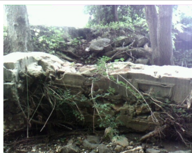
Point # 1035 Location: -76.809364 39.268570 Description: Failed rock wall.
