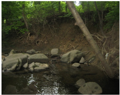
Point # 1048 Location: -76.815140 39.270648 Description: Erosion site. High bank, outside meander.
