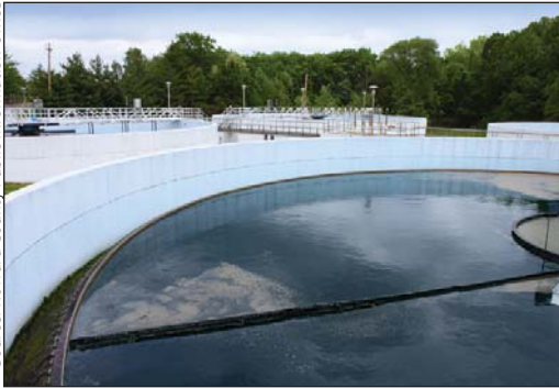
The Little Patuxent Water Reclamation Plant treats wastewater for about 70% of the County served by public sewer.
