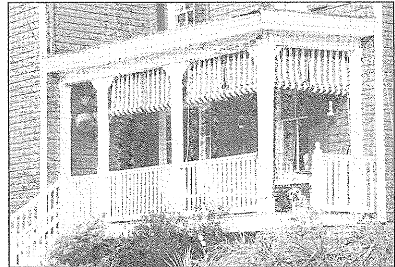
This porch was recently renovated, with new brackets, railings and posts consistent with the character of the older components.
