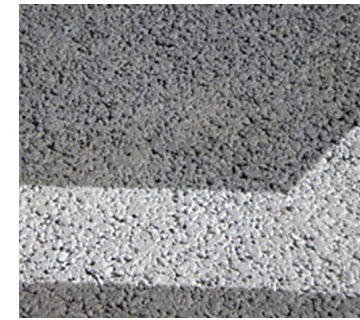
Detail of a porous concrete parking lot at the Robinson Nature Center that absorbs run-off.
