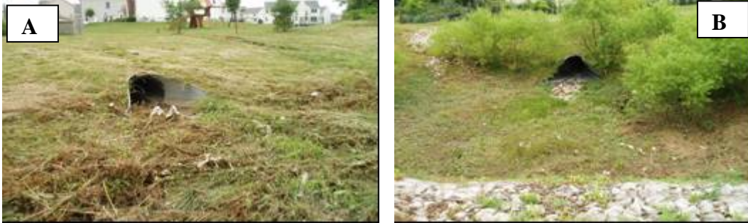
A) View of outfall to dry pond 1. B) View of outfall to dry pond 2.
