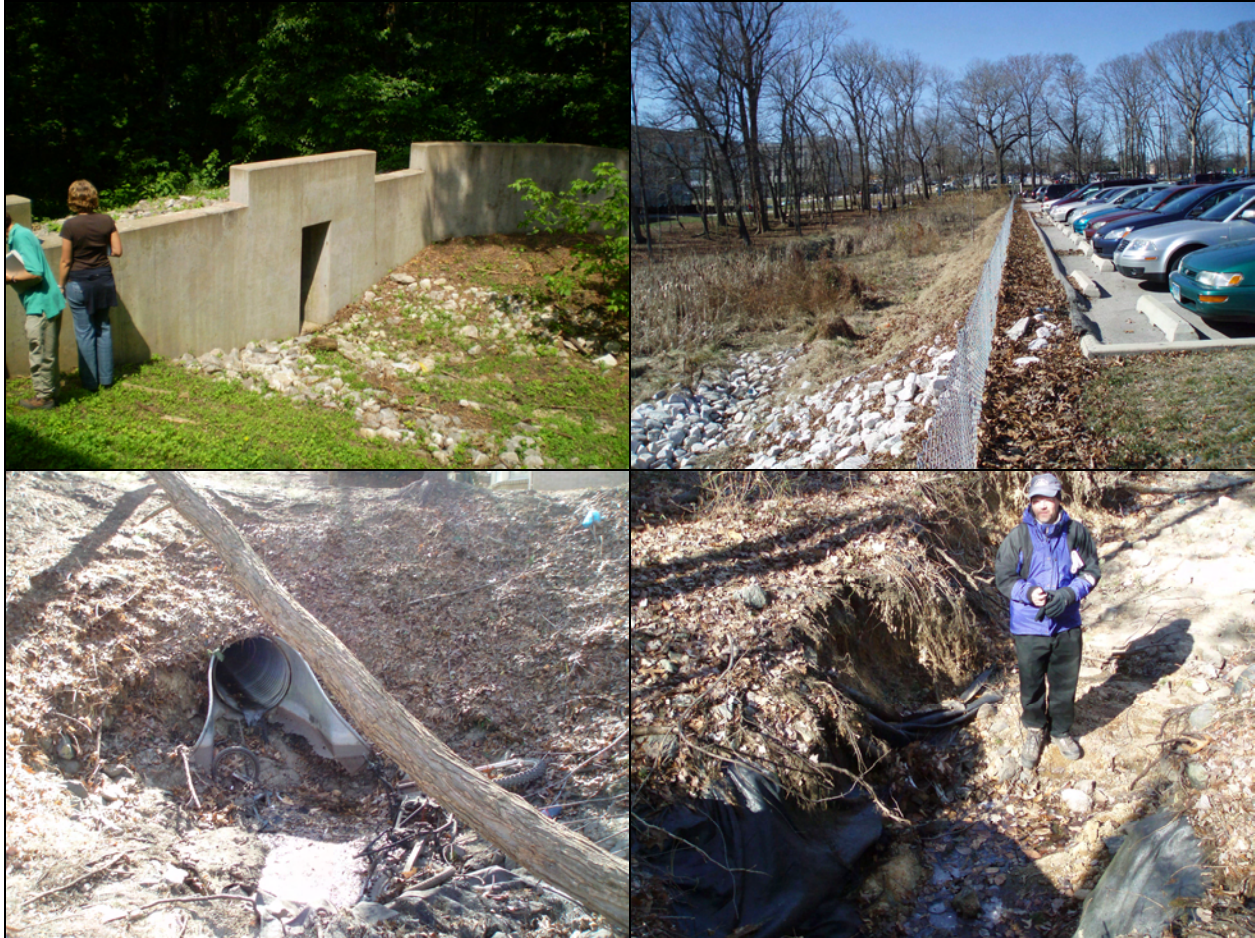
Figure 1-2: Stormwater infrastructure observed throughout the watershed, including: a dry pond that treats runoff from a townhome community (top left); a bioretention practice that treats runoff from a college parking lot (top right); an outfall that discharges unmanaged runoff from an apartment complex (bottom left); and channel erosion resulting from the outfall in the previous photo (bottom right).
