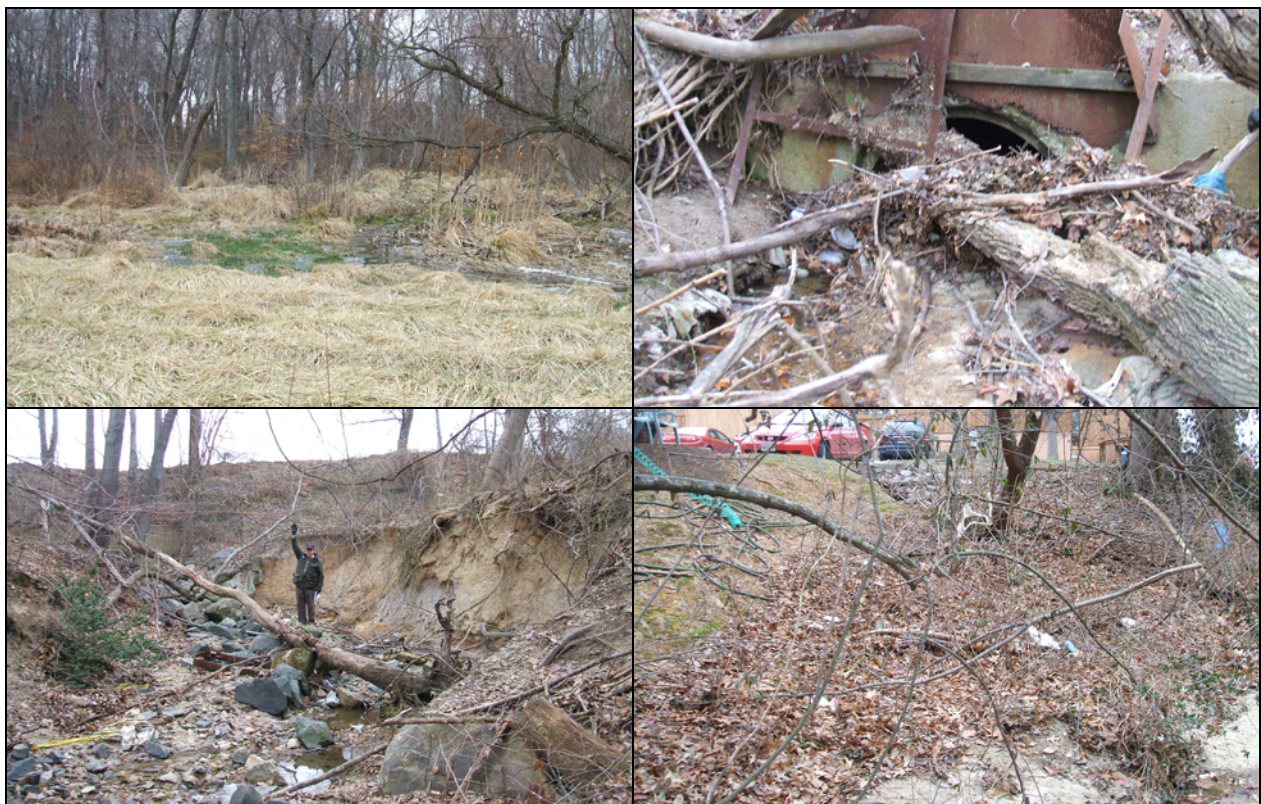
Figure 2-1: Examples of typical impacts observed along Symphony Stream: impacted buffer (top left); a blocked road culvert (top right); severe bank erosion (bottom left); and accumulated trash (bottom right).
