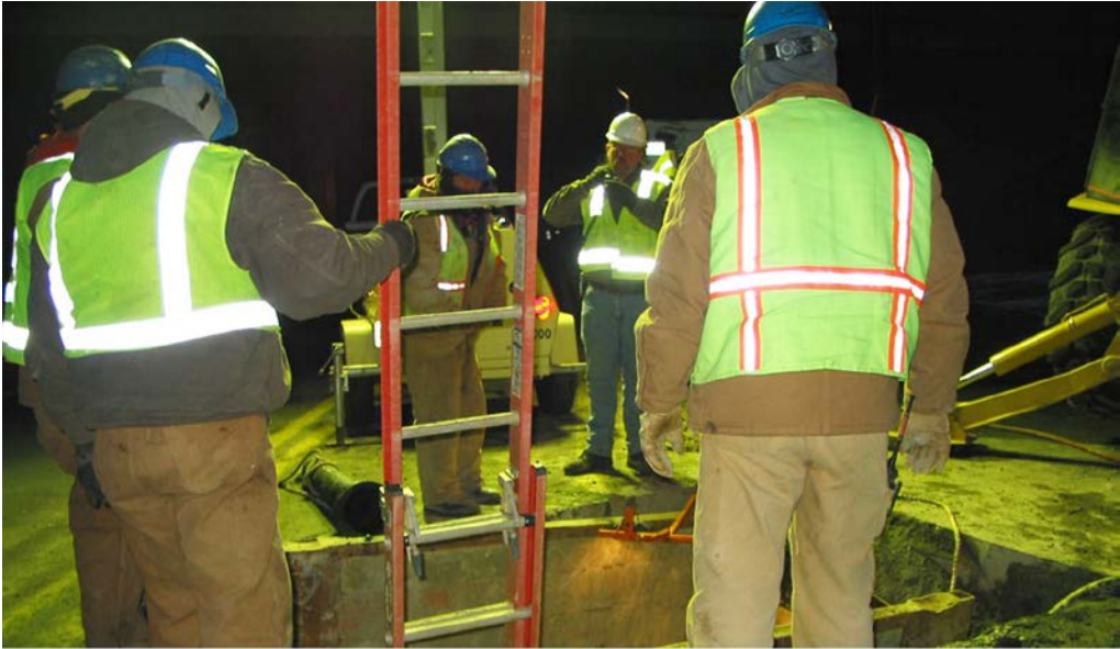
Bureau of Utilities System Maintenance Division maintains Howard County's public water and sewer system ensuring high quality water service and fire protection.
