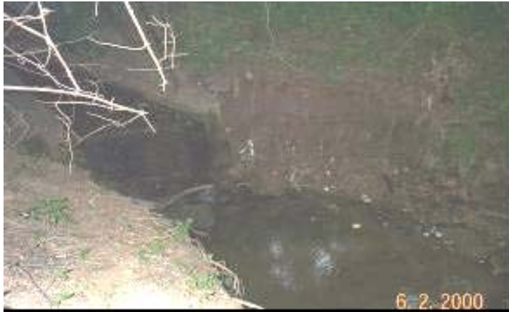
View of eroding bank at the culvert outfall.
