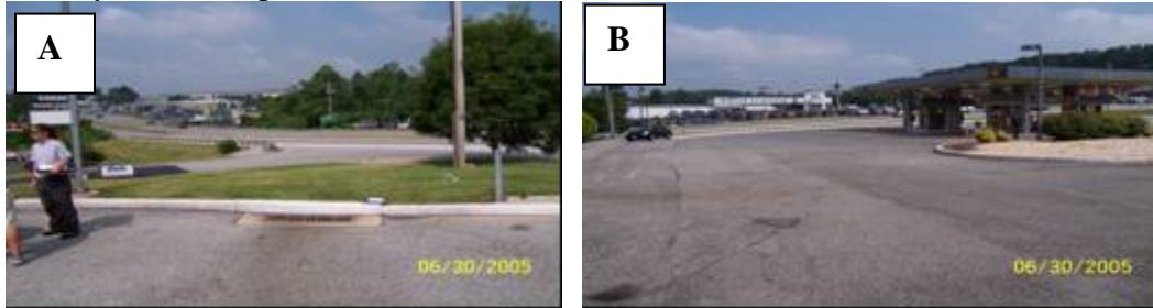
A) View of stormwater drain on parking lot. B) View of gas station where downstream staining may be coming from.
