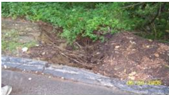
View of eroded curb where runoff bypasses drain inlet and causes erosion.
