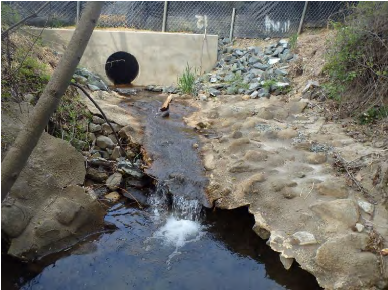
Montevideo Road undercut concrete apron.
