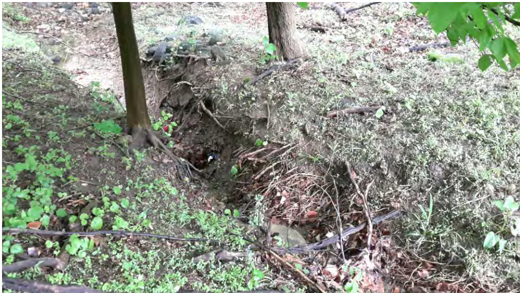
Channel erosion downstream of outfall.
