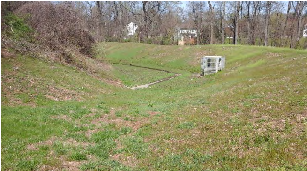
Looking northwest from the access path toward the pond area, concrete inflow channels, riser structure, and embankment.
