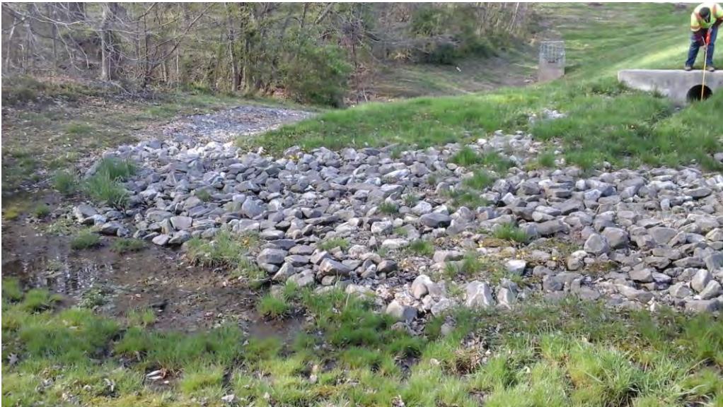
Looking north from the forebay at the inflow, gabion channel, and riser structure.
