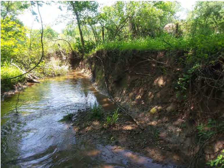
Facing upstream, moderate to severe erosion, 4.5 ft in height with little vegetative cover.
