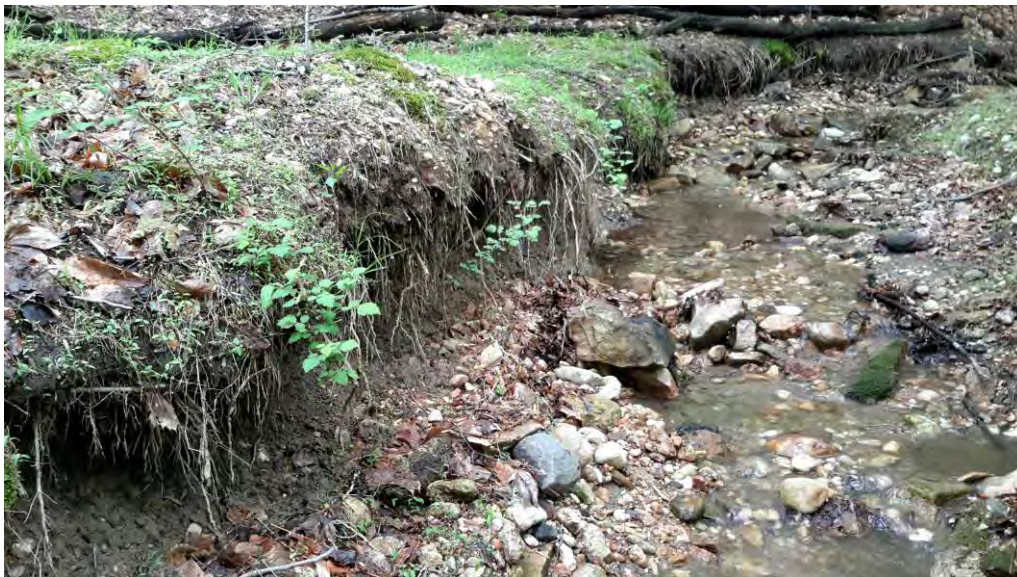
Typical stream bank erosion along the upper portion of the site
