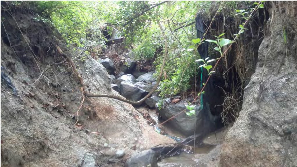
View facing upstream at pipe outfall and eroded outfall channel.
