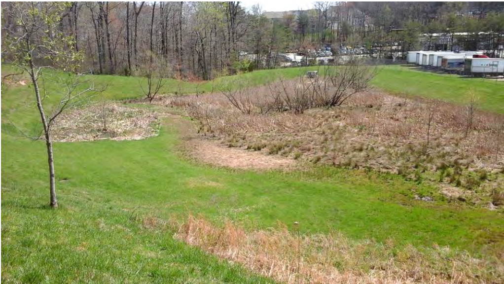
Looking south toward the pond with the inflow, forebay, riser structure, and embankment included in the photo.
