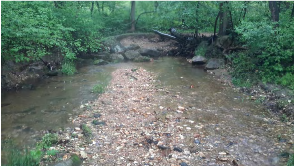
Facing upstream at the sewer crossing showing boulders placed to protect the sewer line
