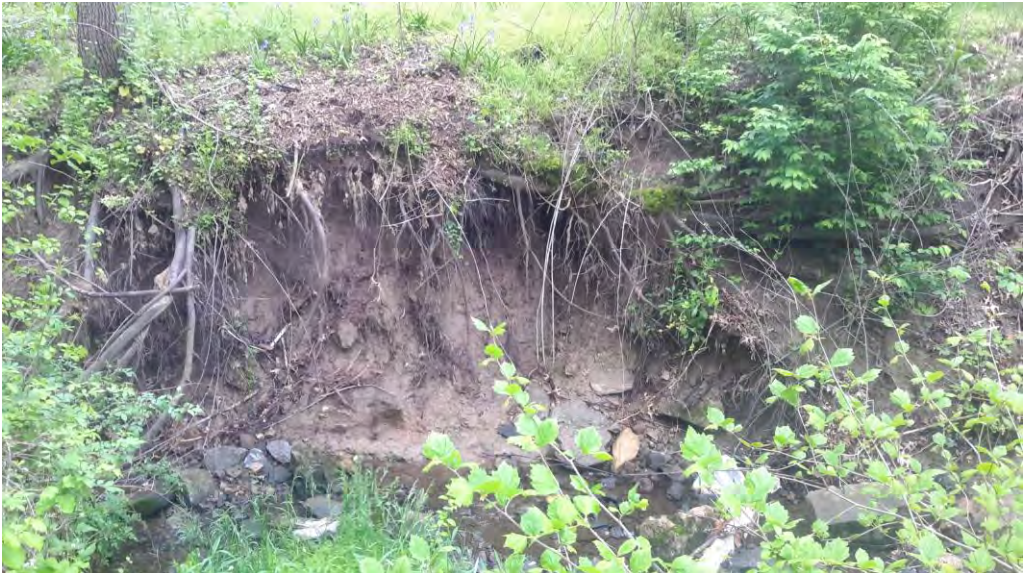
View facing right bank of eroded outfall channel.
