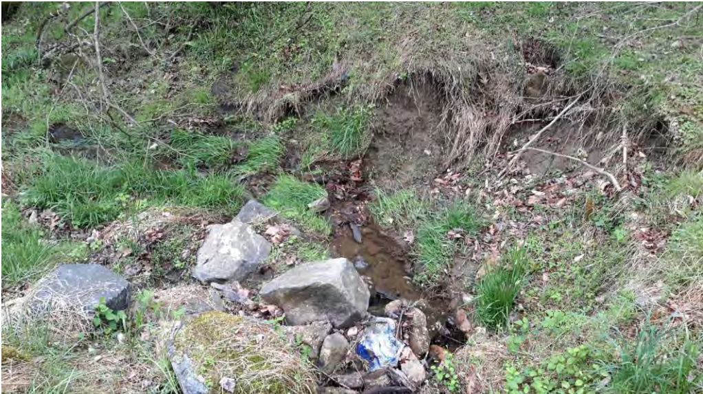
View facing downstream eroded outfall channel.
