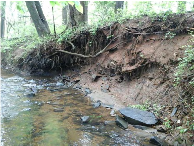
Active severe bank erosion.
