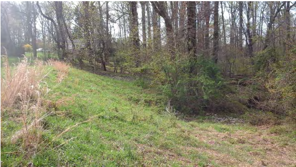
Looking southeast along the downstream side of the embankment at the principal spillway outfall (near riprap) and emergency spillway outfall (far riprap).
