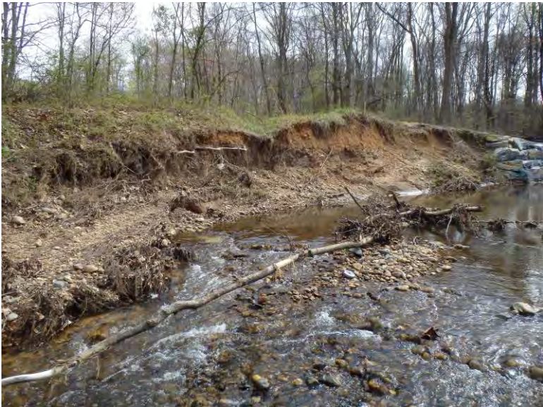
Typical erosion in reach two, upstream and downstream of recent bank stabilization.
