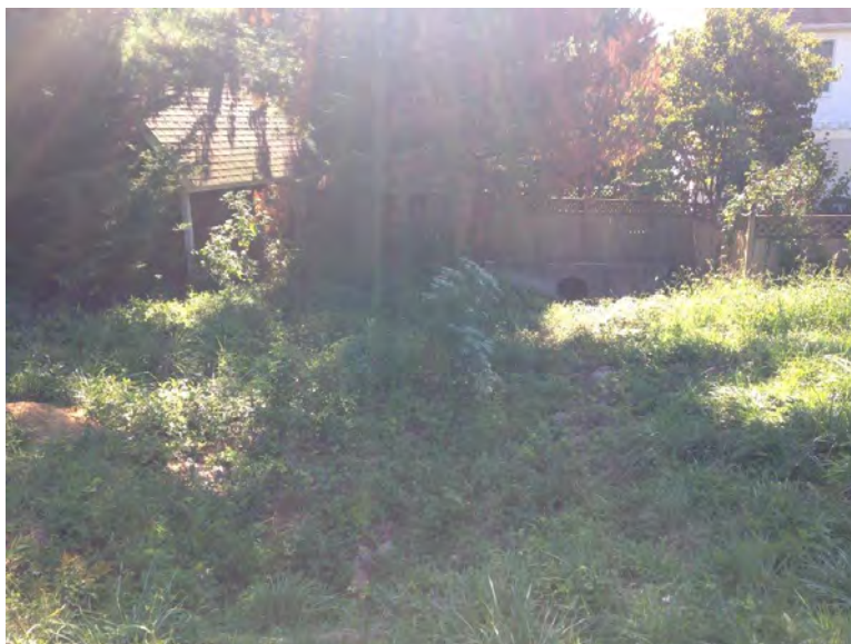
Downstream view to receiving storm drain pipe.
