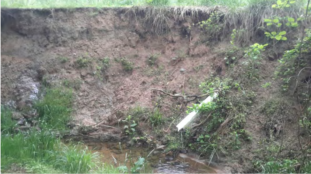
Typical stream bank erosion along the right bank
