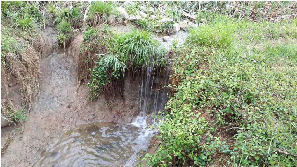
Upper portion of headcut threatening SWM pond outfall
