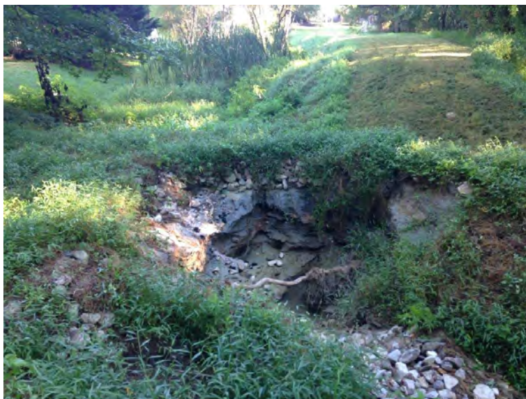
Outfall channel looking upstream to SWM facility. Spillway erosion noted.
