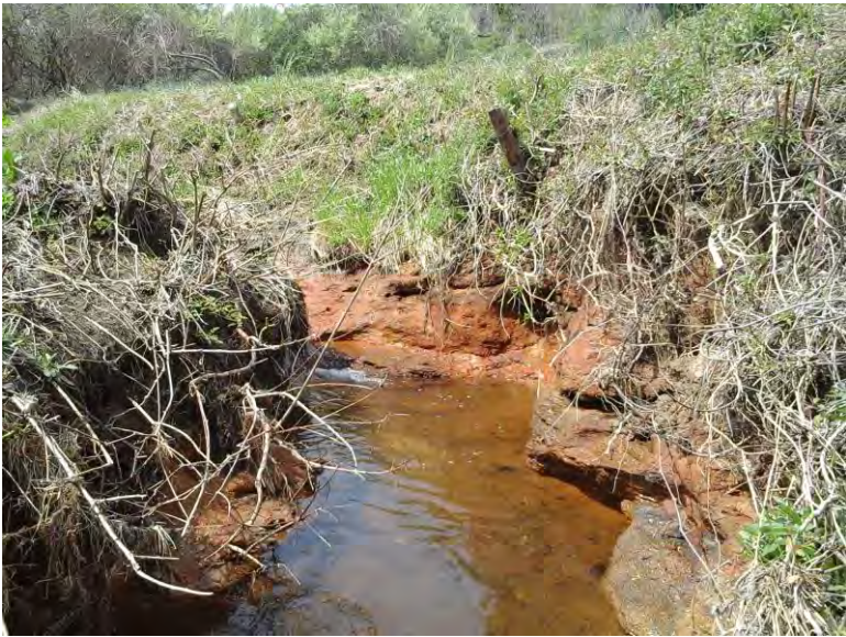
Erosion with bedrock protection.
