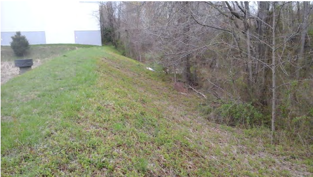
Looking west along the embankment with the riser on the left, outfall on the right, and emergency spillway in the distance.
