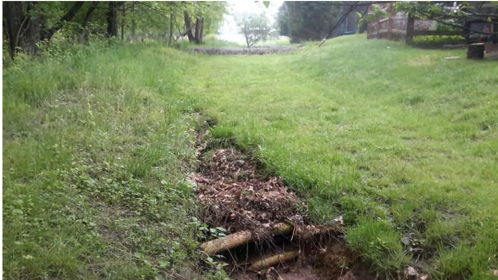
View facing upstream at top of eroded portion of outfall channel.
