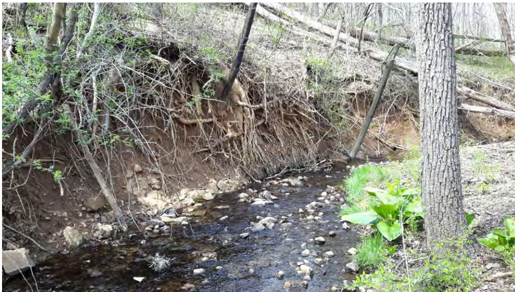
Typical stream bank erosion along the outside of a meander bend
