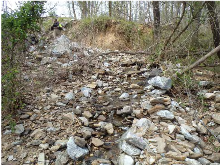
Facing upstream in outfall channel toward left bank erosion.
