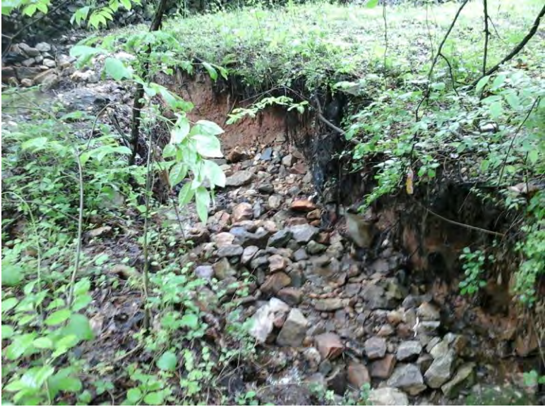
Facing downstream toward outfall channel erosion.
