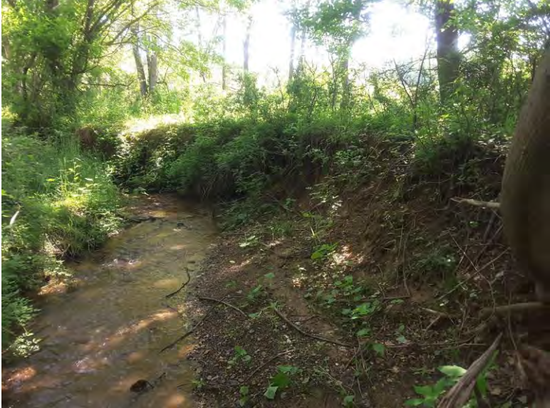
Facing upstream, showing erosion with some slumping visible.
