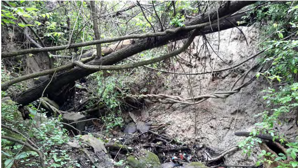
View facing upstream eroded outfall channel.
