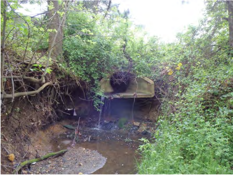
Facing upstream toward destabilized outfall.
