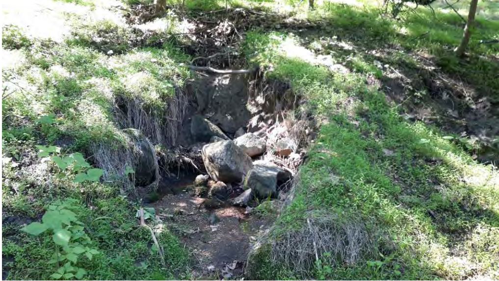
Facing upstream headcut near midpoint of site
