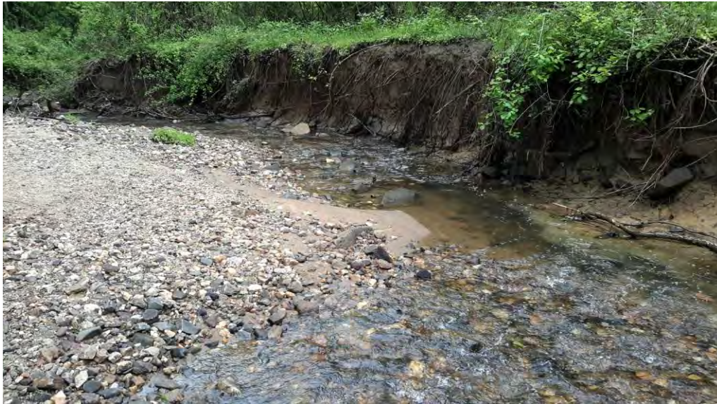
Typical erosion along the left bank
