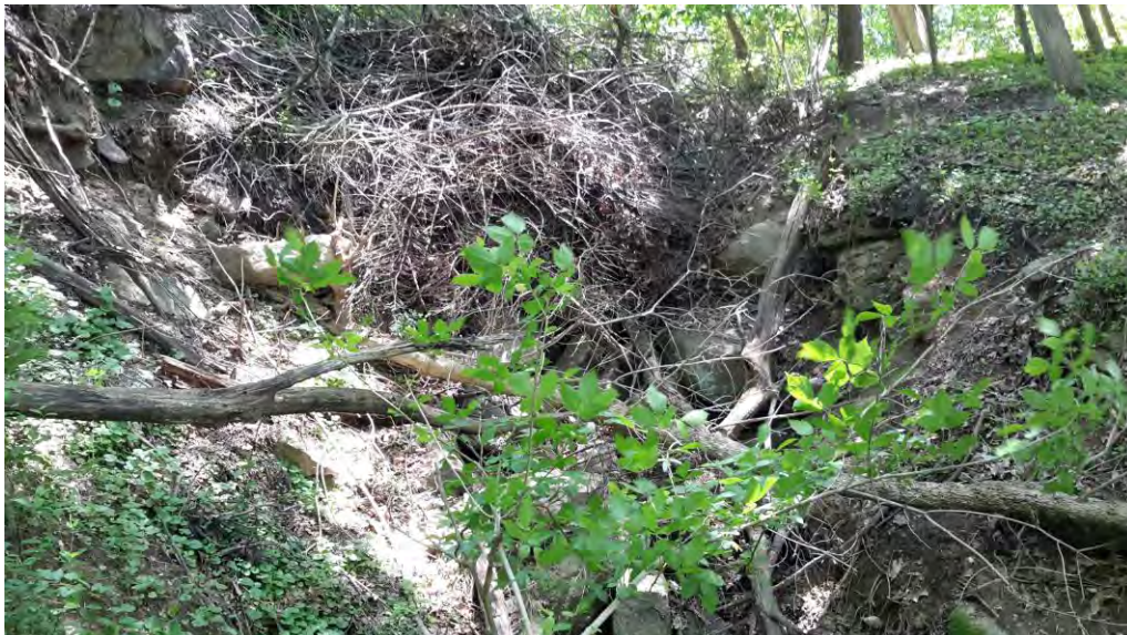
View facing upstream eroded channel.
