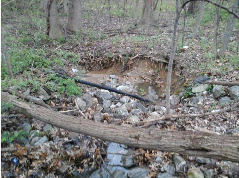
Facing downstream in outfall channel toward right bank erosion.
