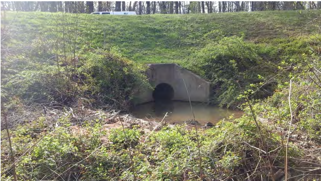
Looking west toward the outfall from the area where erosion and headcuts begin.
