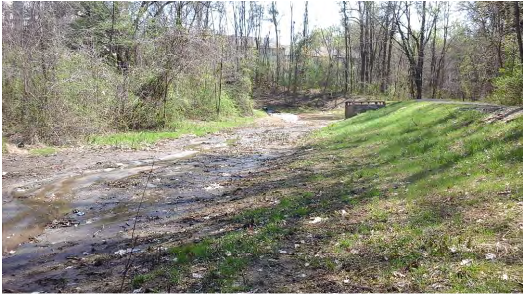
Looking southeast toward the riser structure from the center of the pond.
