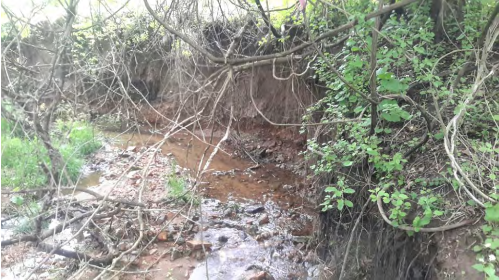
Typical stream bank erosion along the left bank
