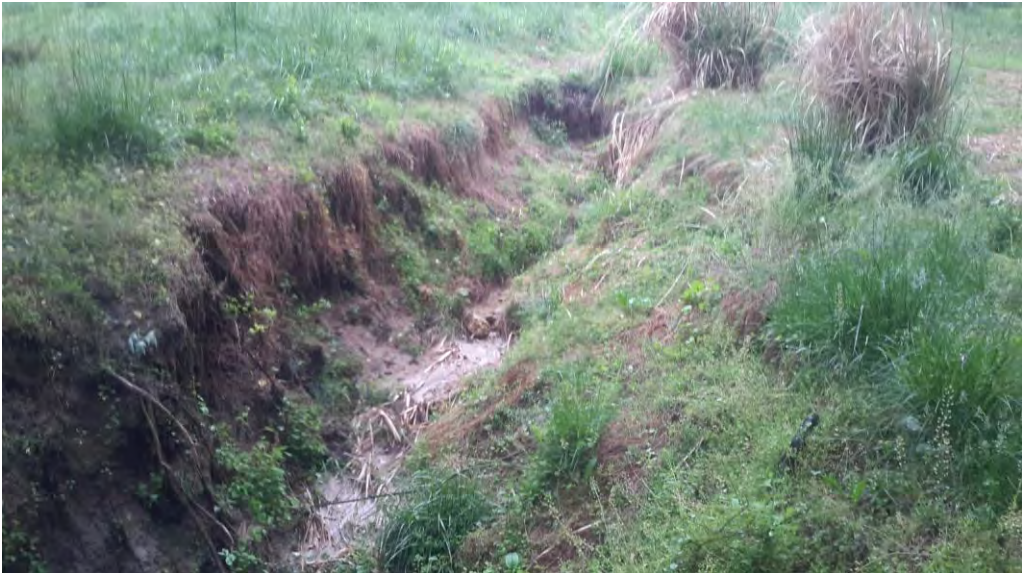
View of erosion looking upstream.
