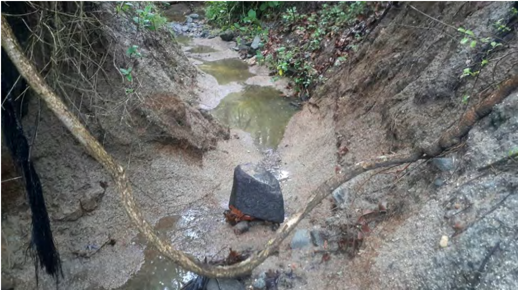
View facing downstream of eroded outfall channel.
