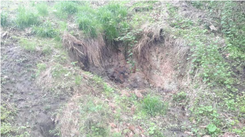
View facing upstream of outfall erosion on western channel.
