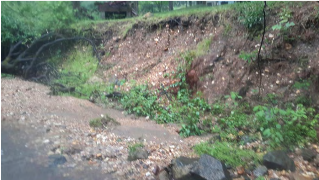
Typical stream bank erosion in the lower portion of the site
