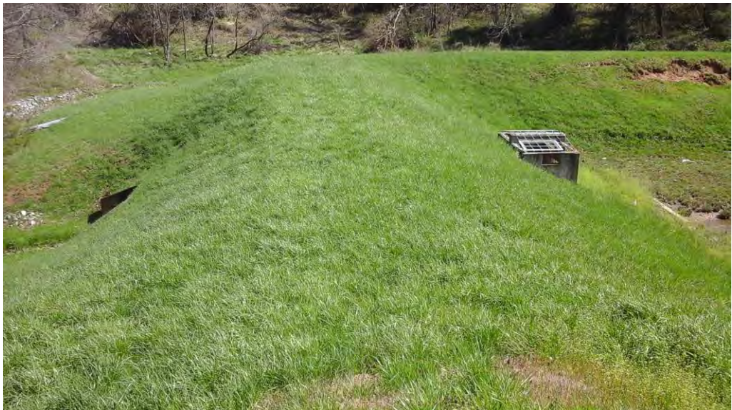
Looking southeast along the embankment toward the riser structure and outfall from the top of the embankment near the parking lot and access gate.
