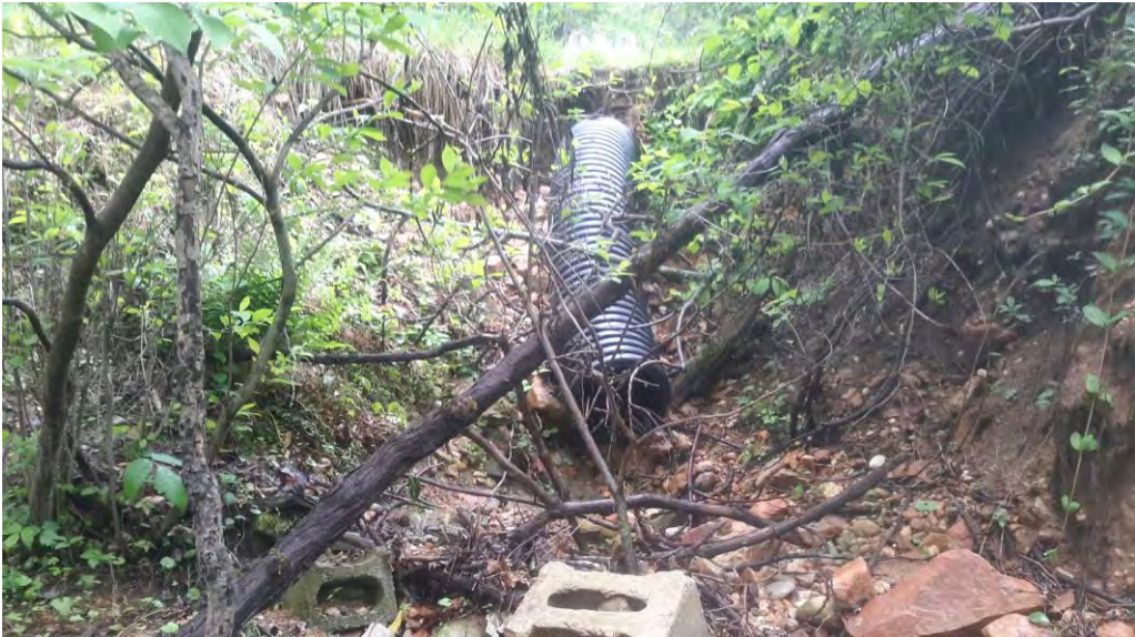
View facing upstream of exposed outfall pipe and eroded channel.
