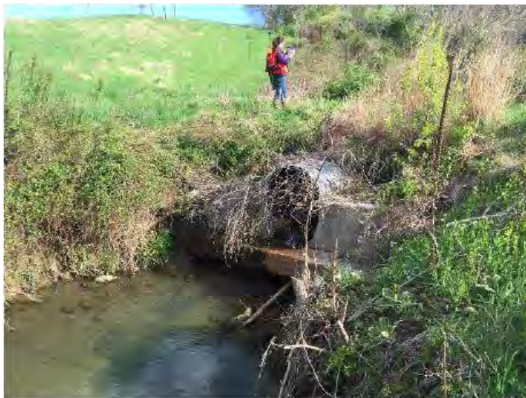
Looking upstream at perched culvert where tributary enters the concept reach (photo courtesy of Century Eng.)
