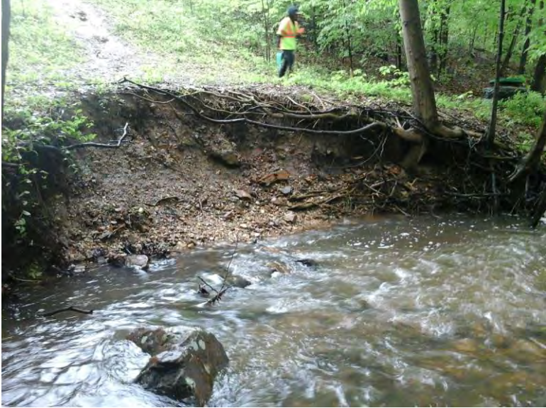
Erosion which may threaten sewer if untreated.
