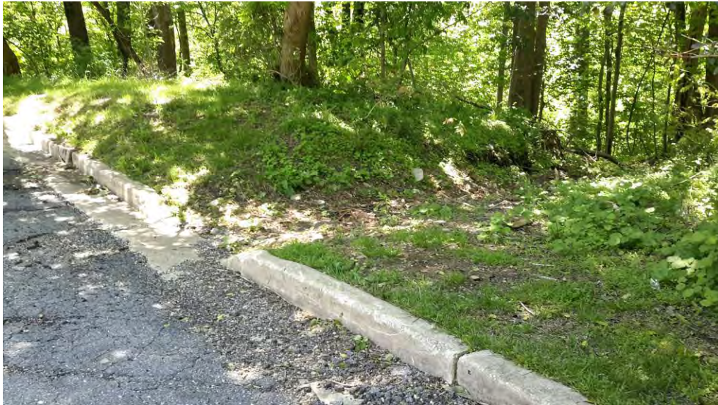
View of curb cut in parking lot at top of eroded channel.
