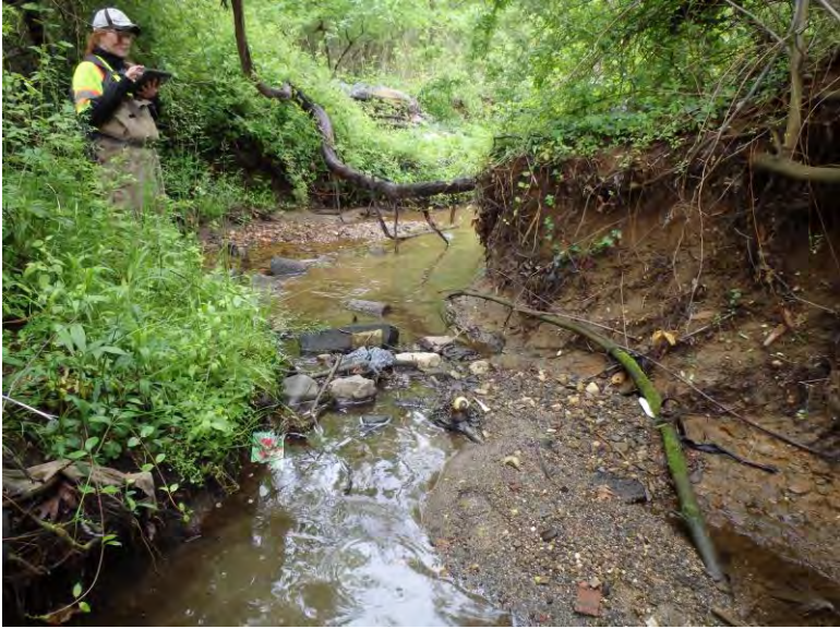
Facing downstream toward erosion in outfall channel and tributary confluence.
