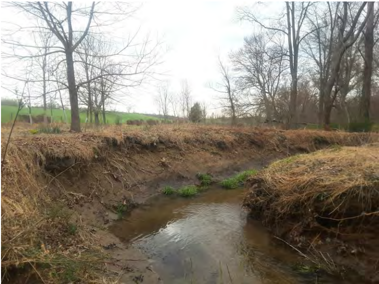
Facing downstream, at a tight bend, displaying the poor bank protection, erosion, and insufficient buffer.
