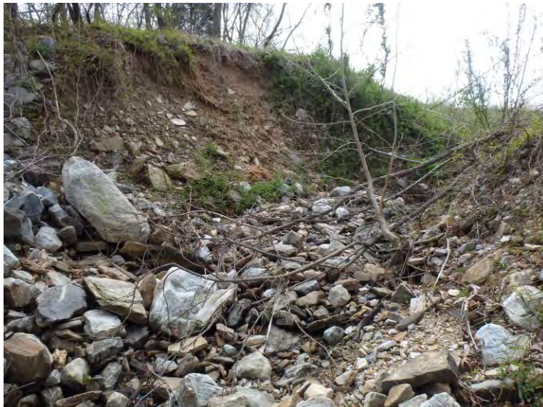
Facing upstream in outfall channel toward right bank erosion.
