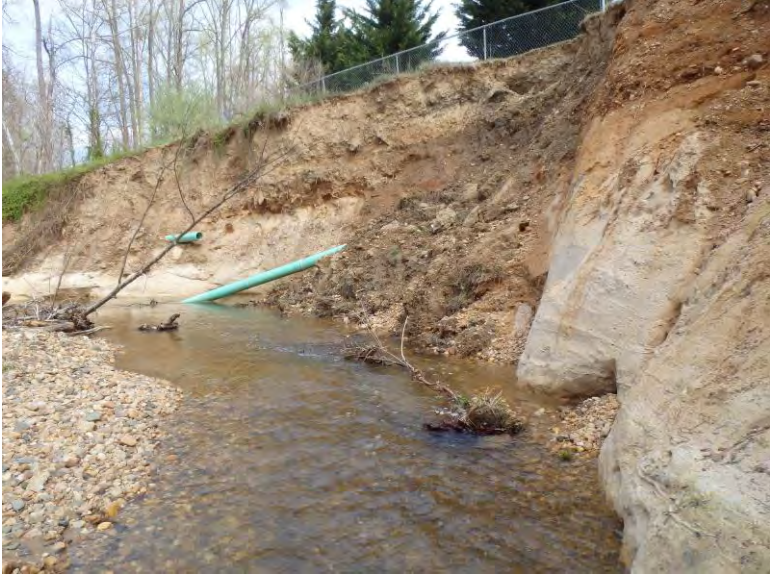
Reach one erosion threatening stormwater pond embankment.
