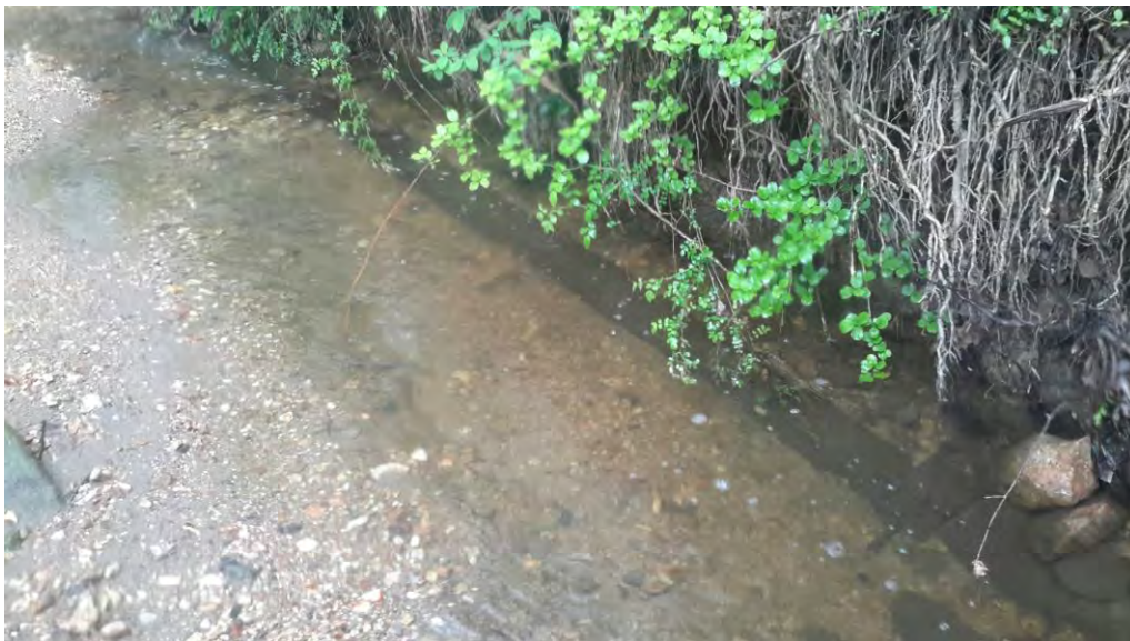
Exposed sewer line in the channel bed
