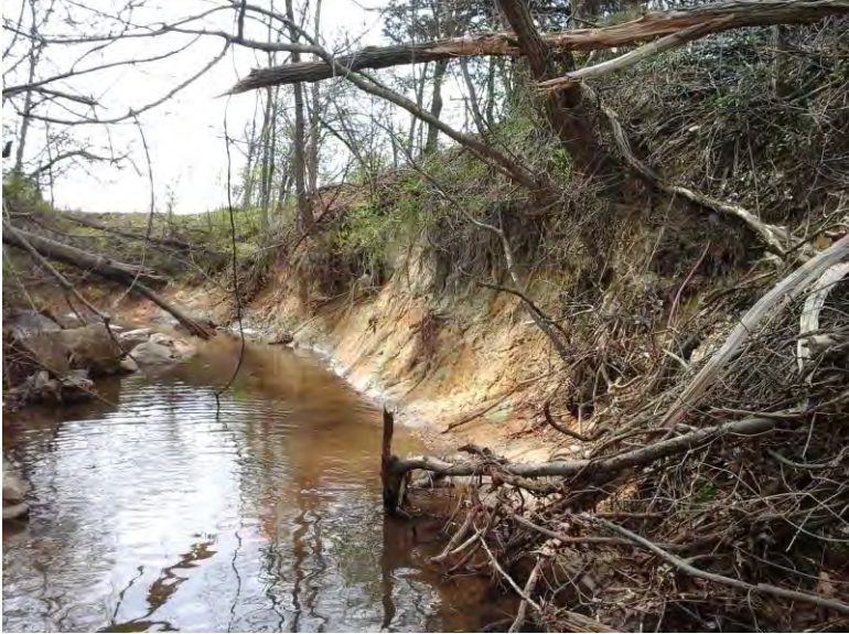
Typical erosion threatening private road.
