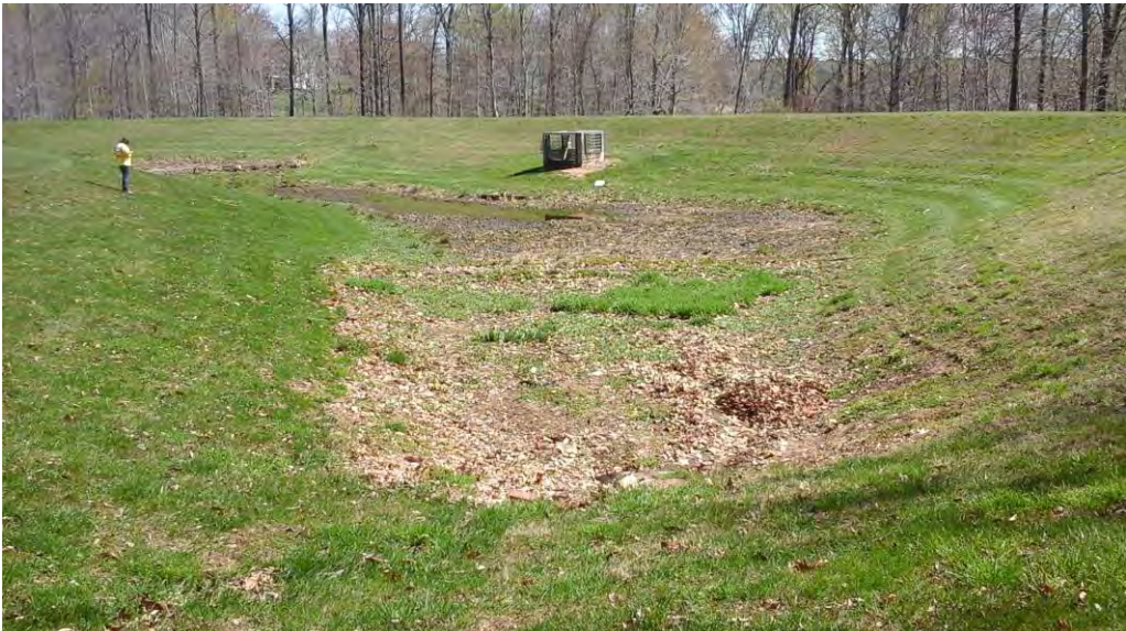
Looking north from the south inflow toward the pond area, riser, and embankment.
