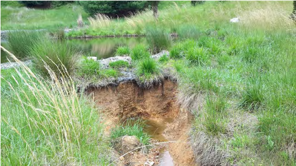
View facing upstream at headcut below gabion weir.
