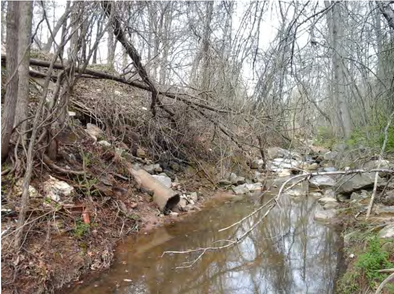
Riprap stabilization and disconnected outfall end section.
