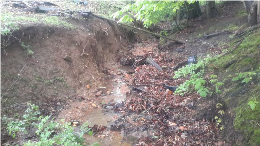
Typical stream bank erosion in the upper portion of the site
