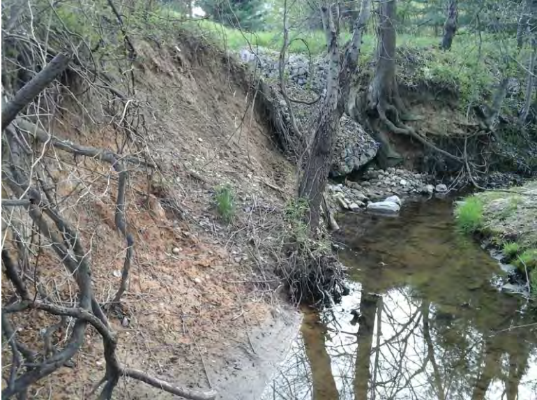
Severe bank erosion and gabion slumping.
