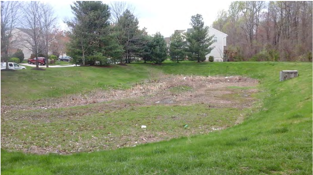
Looking northwest at the pond area with the inflows and forebay on the left and riser structure and embankment on the right.
