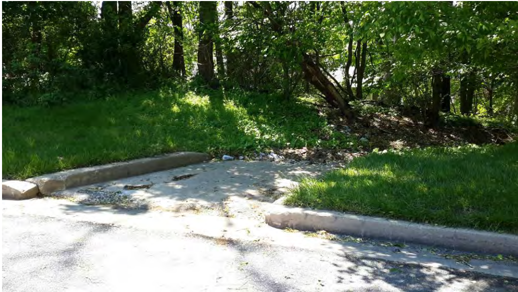
View of curb cut in parking lot at top of eroded channel.
