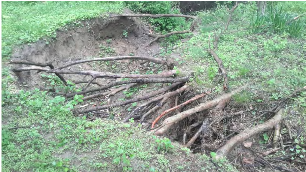
View facing downstream of headcut in eroded outfall channel.
