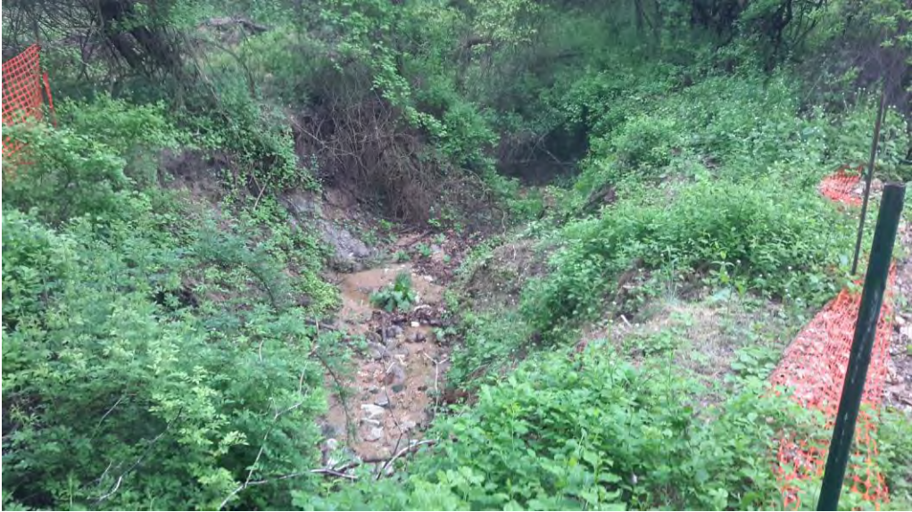
View of erosion facing downstream from outfall.
