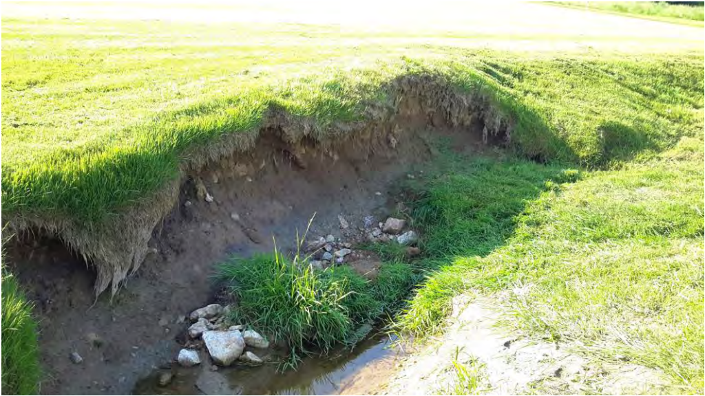
Typical stream erosion along the site
