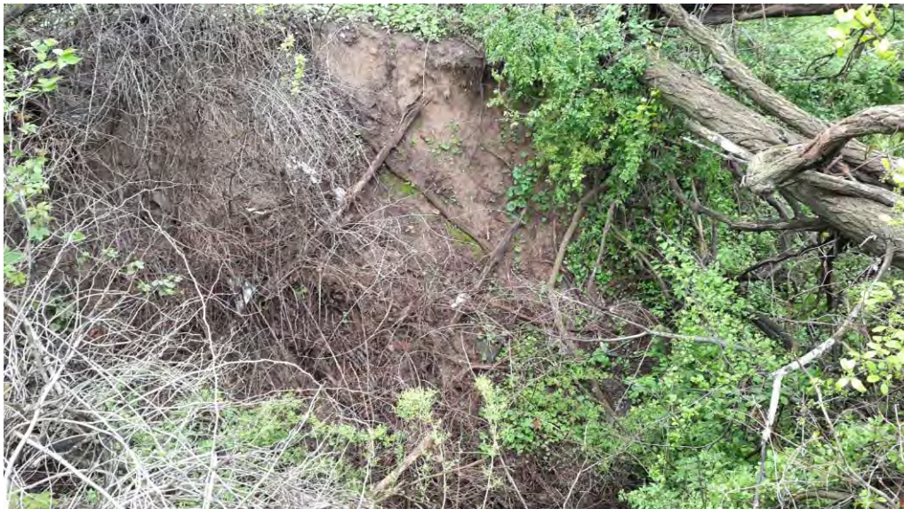
View facing left bank of eroded outfall channel.
