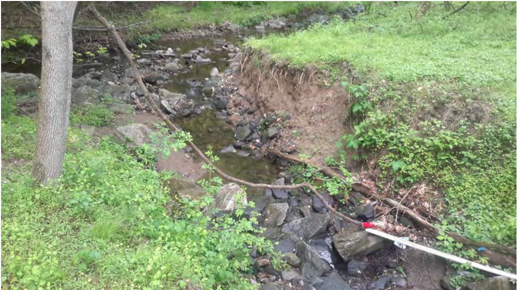
View facing downstream in eroded outfall channel.
