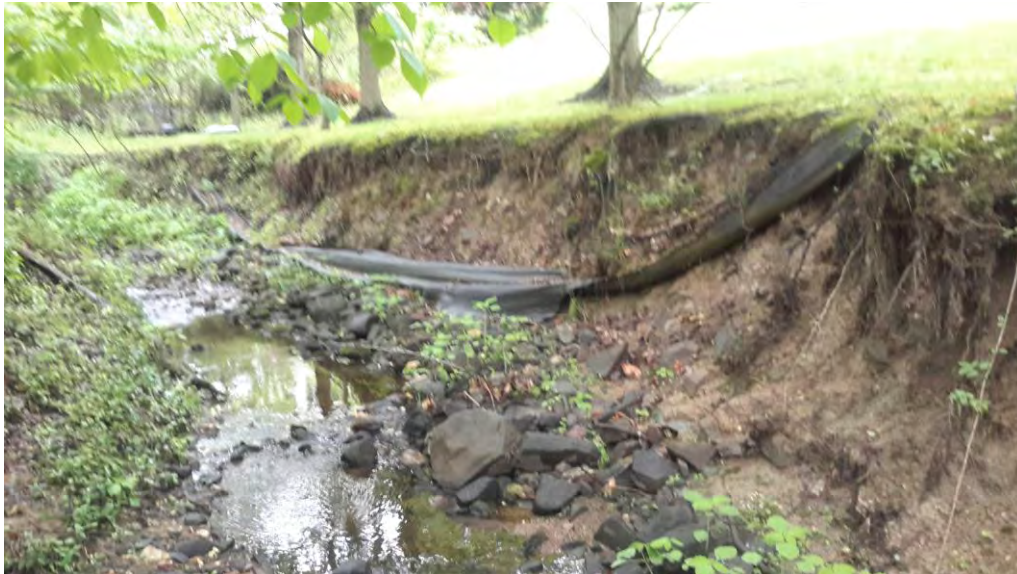
Typical stream bank erosion at this site
