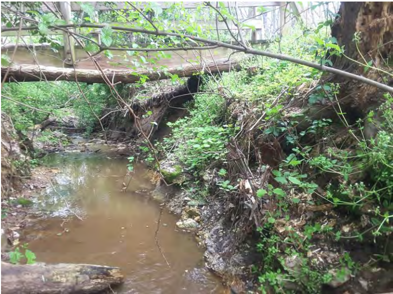
Photo facing upstream at left bank erosion associated with the bridge crossing. Stable restoration tie in point would be downstream of this location.
