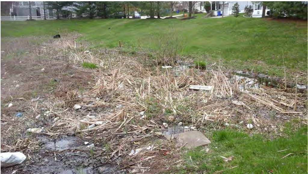
Looking southeast at the forebay from the inflow on the western side of the pond.
