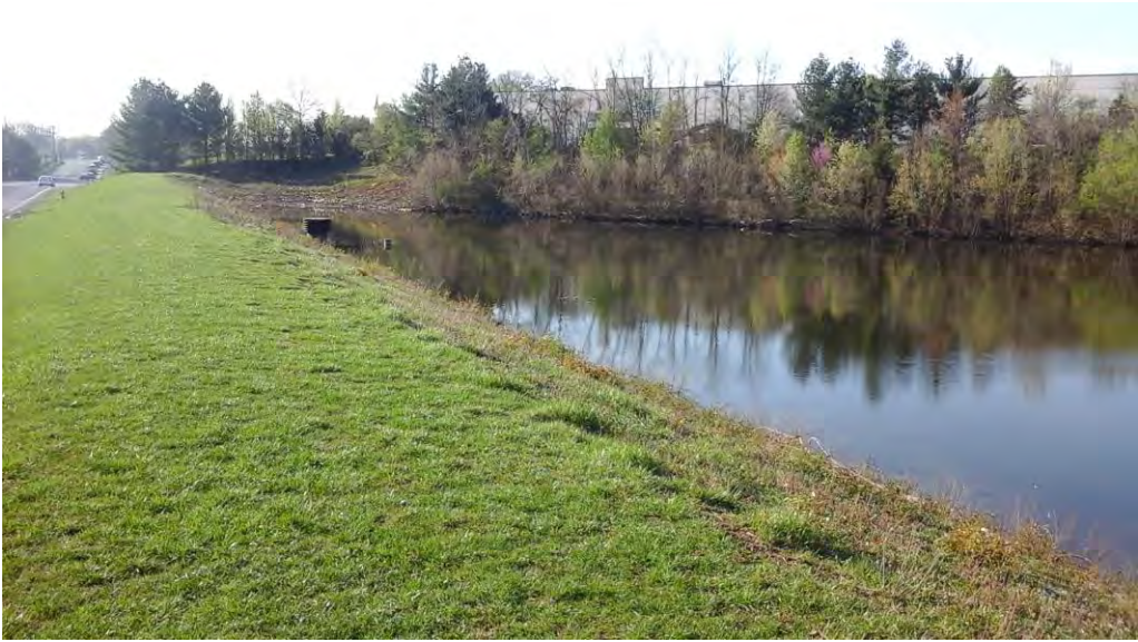
Looking southeast along the embankment toward the riser structure and emergency spillway.
