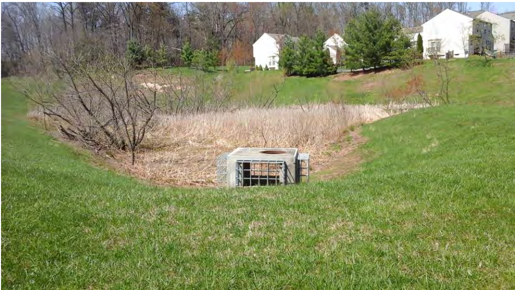
Looking north toward the riser and pond area from the embankment with areas of erosion and the access in the distance.
