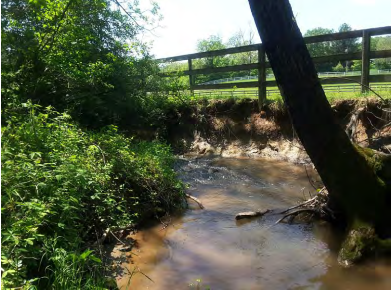
Facing the left bank, pasture fencing on the 14010 Forsythe Rd property at risk from erosion.
