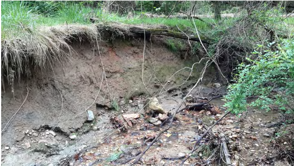
Typical stream bank erosion along the lower portion of the site
