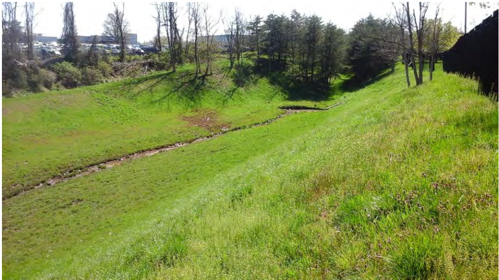
Looking southwest toward the pond inflow from the embankment near the parking lot.
