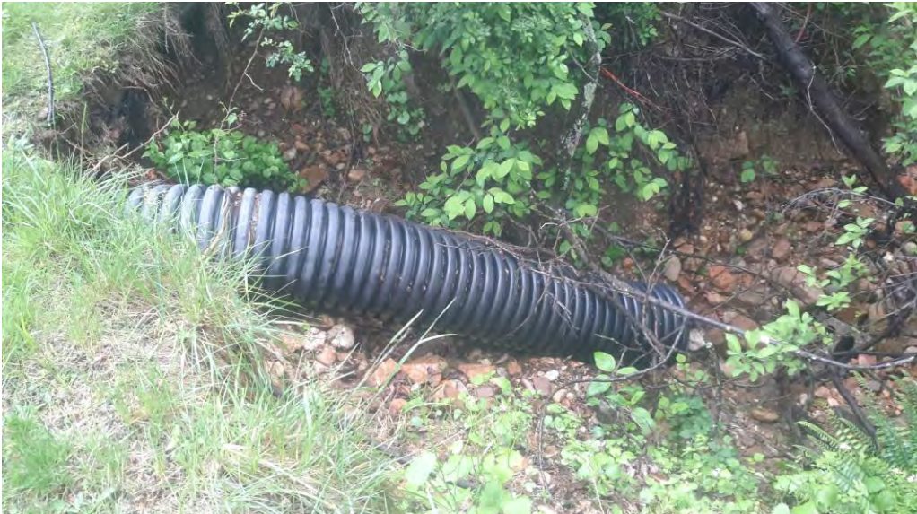
View facing downstream of exposed outfall pipe and eroded channel.
