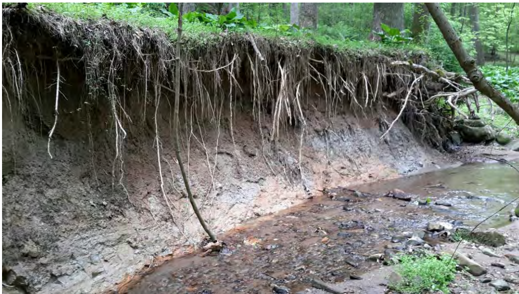
Typical stream bank erosion on the right bank
