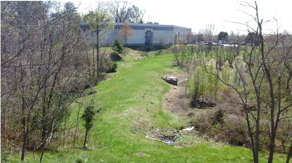
Looking southeast toward the embankment and riser structure from the building parking lot.
