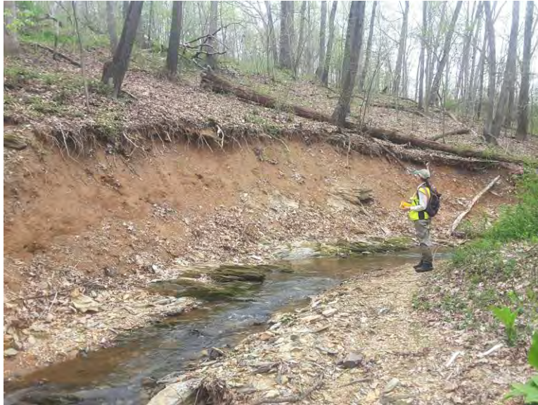
Photo facing upstream at 14 ft. high right bank with bedrock toe protection/stabilization.
