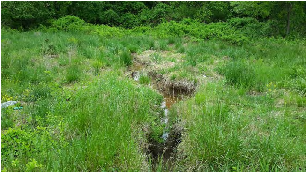
View facing downstream of eroded outfall channel.
