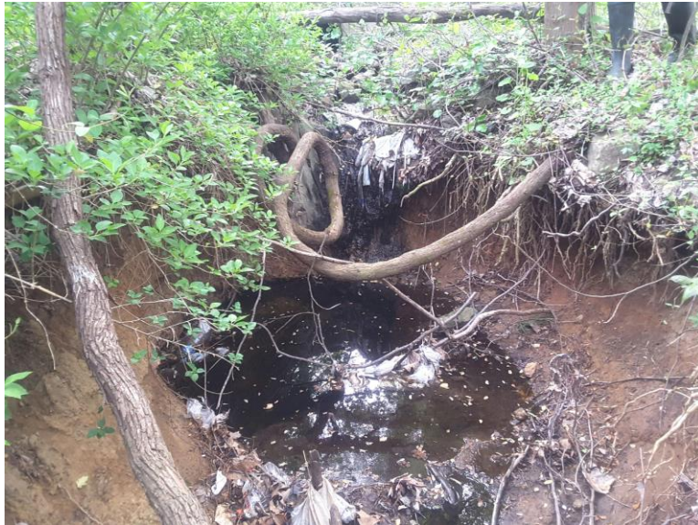
Photo facing upstream at the existing 5 ft. headcut caused from outfall PRU-OF-F306A.
