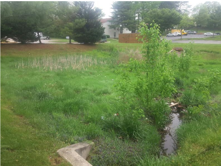
Overview of the facility, including inlet headwall and outlet riser structure, looking northeast
