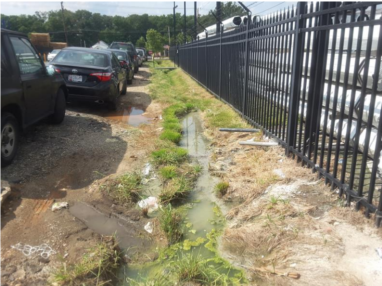
Overview of existing swale showing examples of drainage issues
