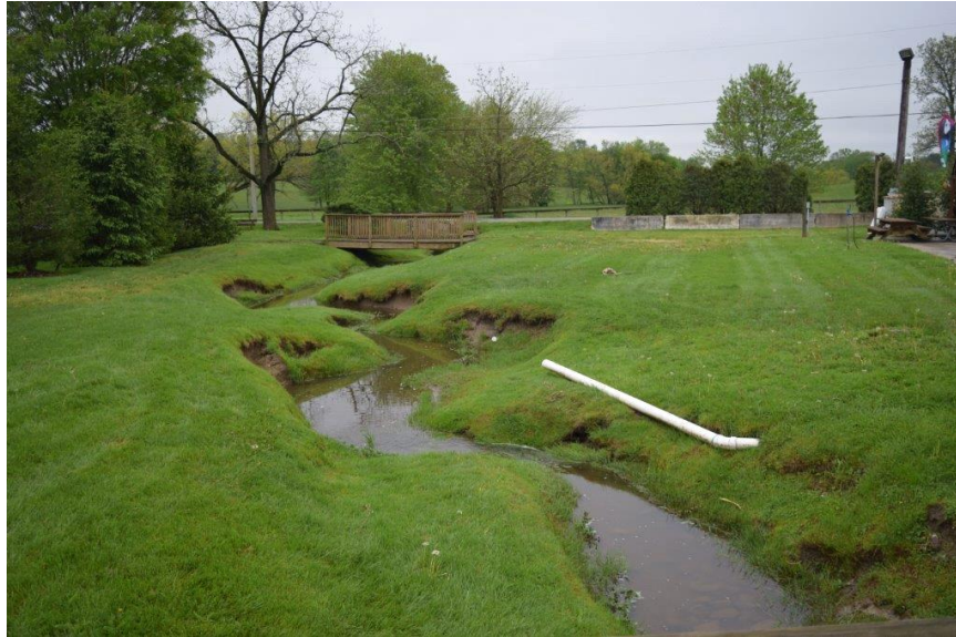
Along the northern property, tight meander bends with eroding and sloughing banks. Several pipes discharge roof runoff along the stream banks.
