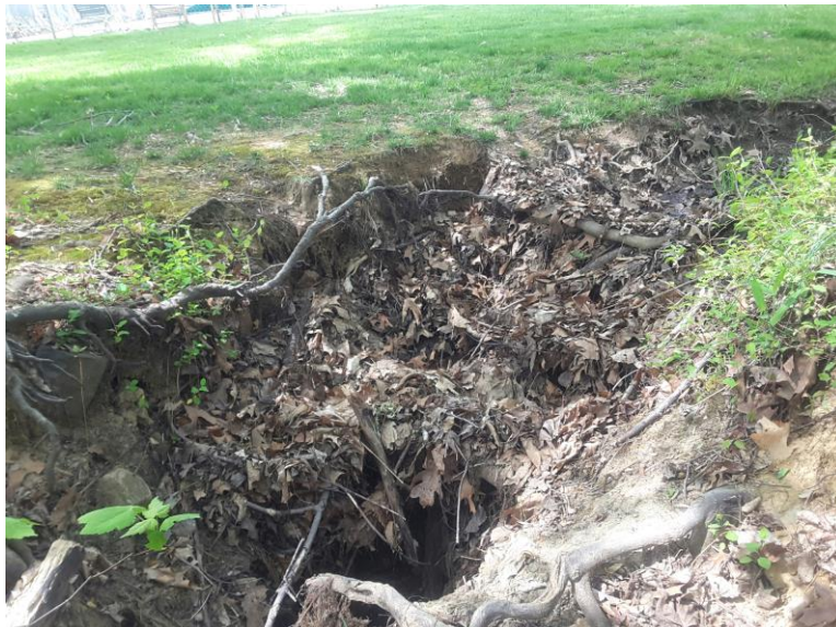
Photo facing upstream at the existing 3.5 ft. headcut caused from outfall PRU-OF-F306B.
