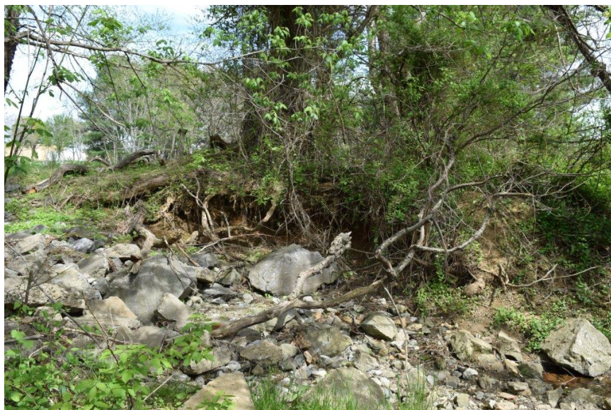
Active headcut requiring stabilization from end of concrete drainage channel (just out of photo to the left) to confluence with stream (bottom right).
