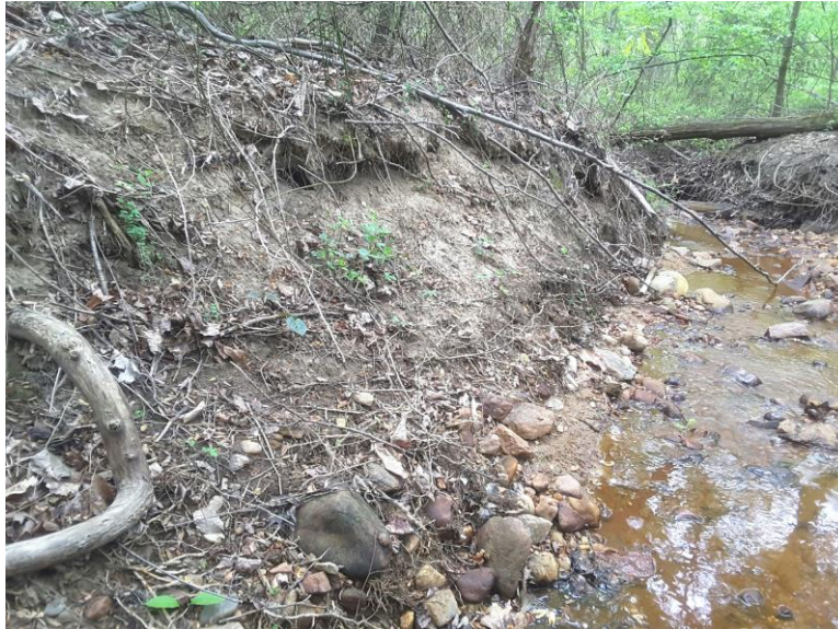
Photo facing downstream of bank erosion along the right bank.
