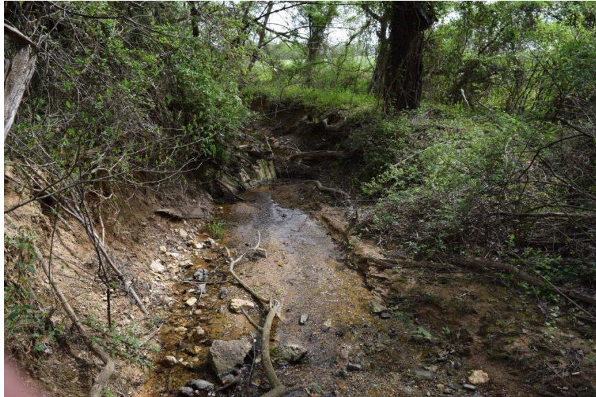
Bank erosion and accumulation of trees and brush looking downstream along school property.
