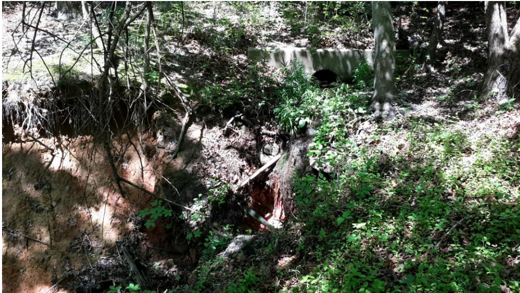
View of headcut at outfall pipe.
