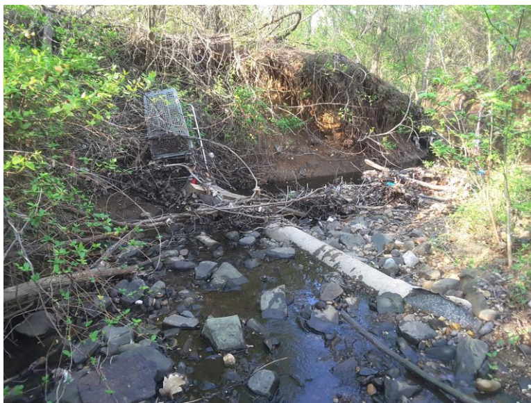
Photo facing downstream showing high left bank at tight meandering bend. Photo shows exposed sewer line and trash in-stream.
