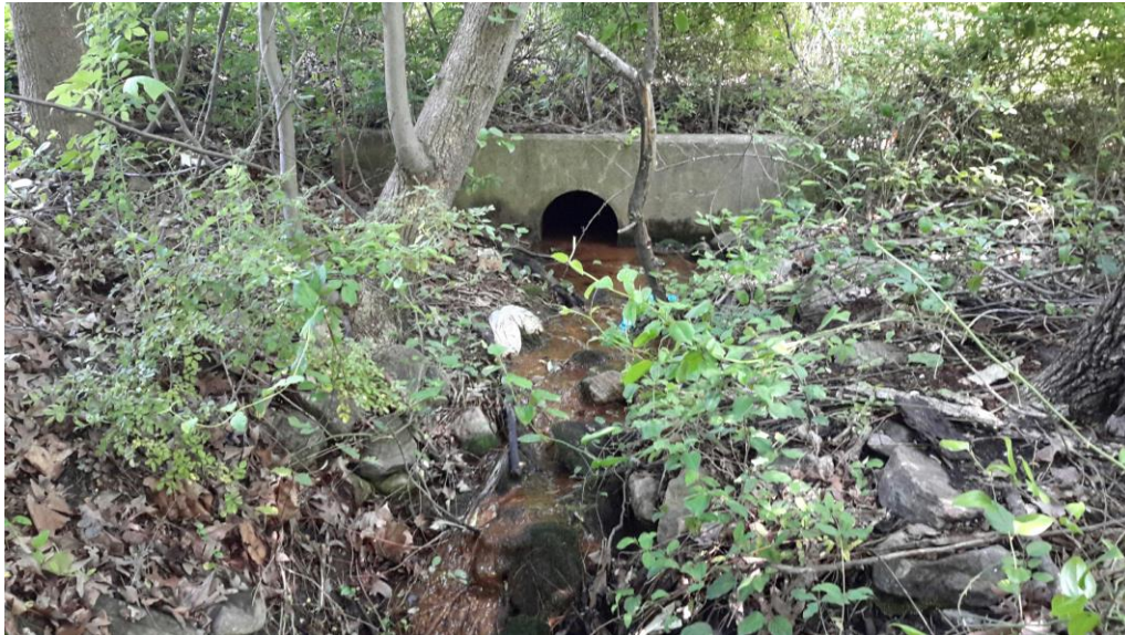
View of headcut at outfall pipe.
