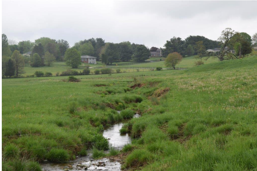
Typical stream conditions across eastern fields from culvert under AE Mullnix Rd. Bank erosion estimated to be 4 ft. or more in height at some locations.
