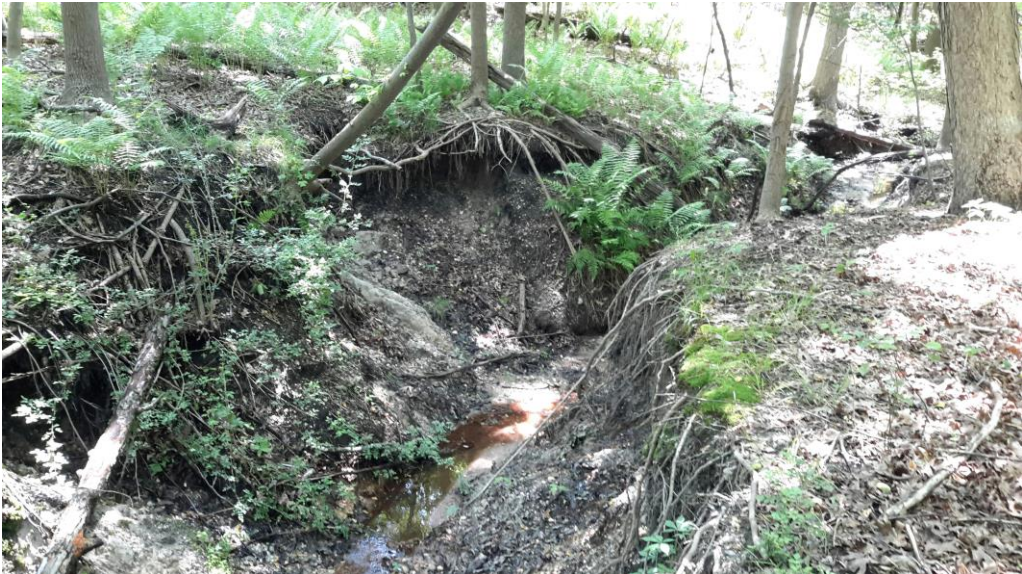
Facing downstream at typical left bank erosion
