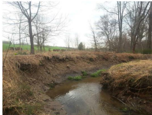
Facing downstream, at a tight bend, displaying the poor bank protection, erosion, and insufficient buffer.
