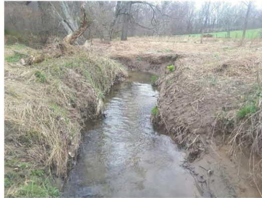
Facing upstream, displaying the poor bank protection and erosion.
