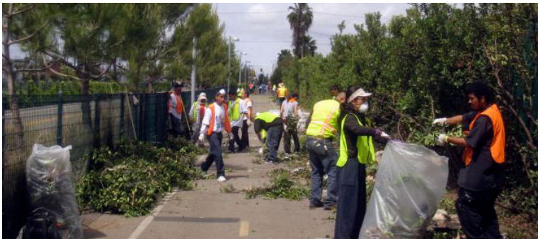
Example of Trail Cleanup Effort Source: Los Angeles County Metropolitan Transportation Authority
