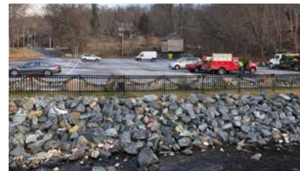
Figure 72: Boulders and Fencing Were Placed Between Lot F and the Stream Channel as Part of the Parking Lot's 2019 Reconfiguration.
