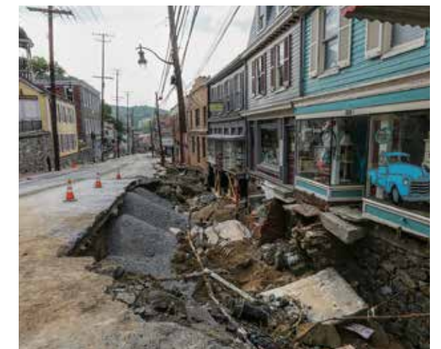
Figure 32: Sidewalk and Utility Damage at 8247 Main Street Immediately following the 2016 flood
