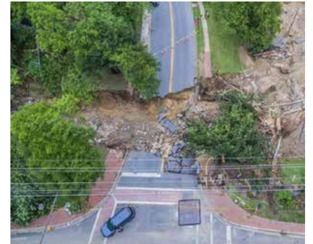
Figure 46: Ellicott Mills Drive Culvert After the 2018 Flood
