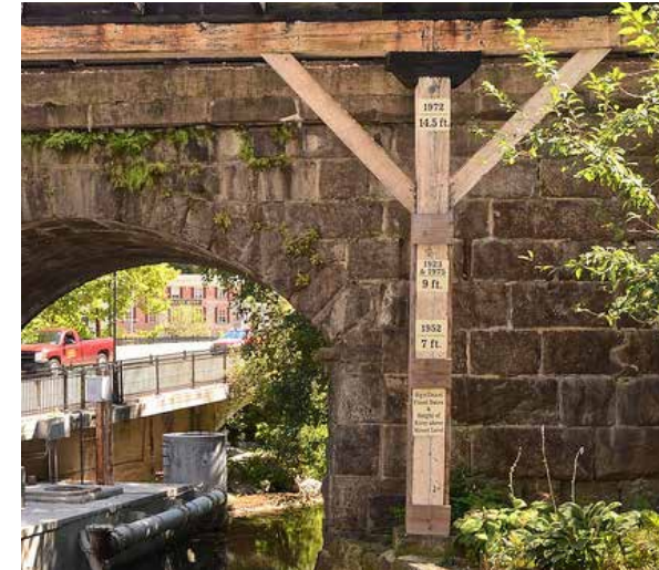
Figure 45: High Water Mark in Ellicott City on the Oliver Viaduct (Pre 2016 Flood), Credit Frank Monaldo
