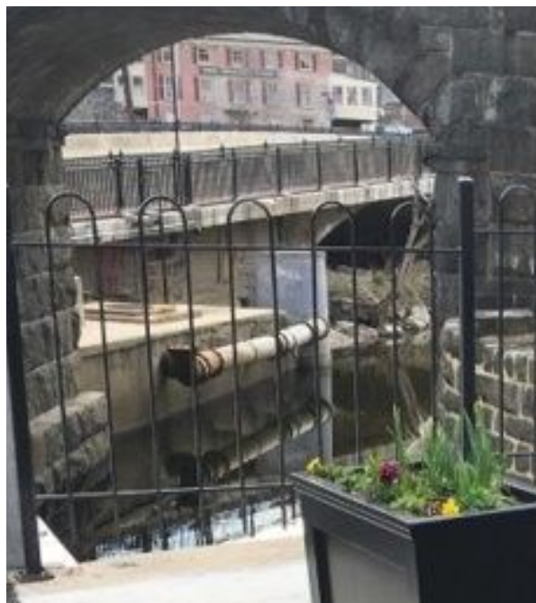
Figure 135: The Oliver Viaduct’s Narrow Opening Restricts Flood Conveyance in Lower Main
