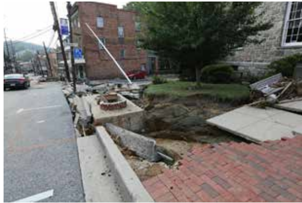
Figure 96: Damage to Brick Paving after the 2018 Flood
