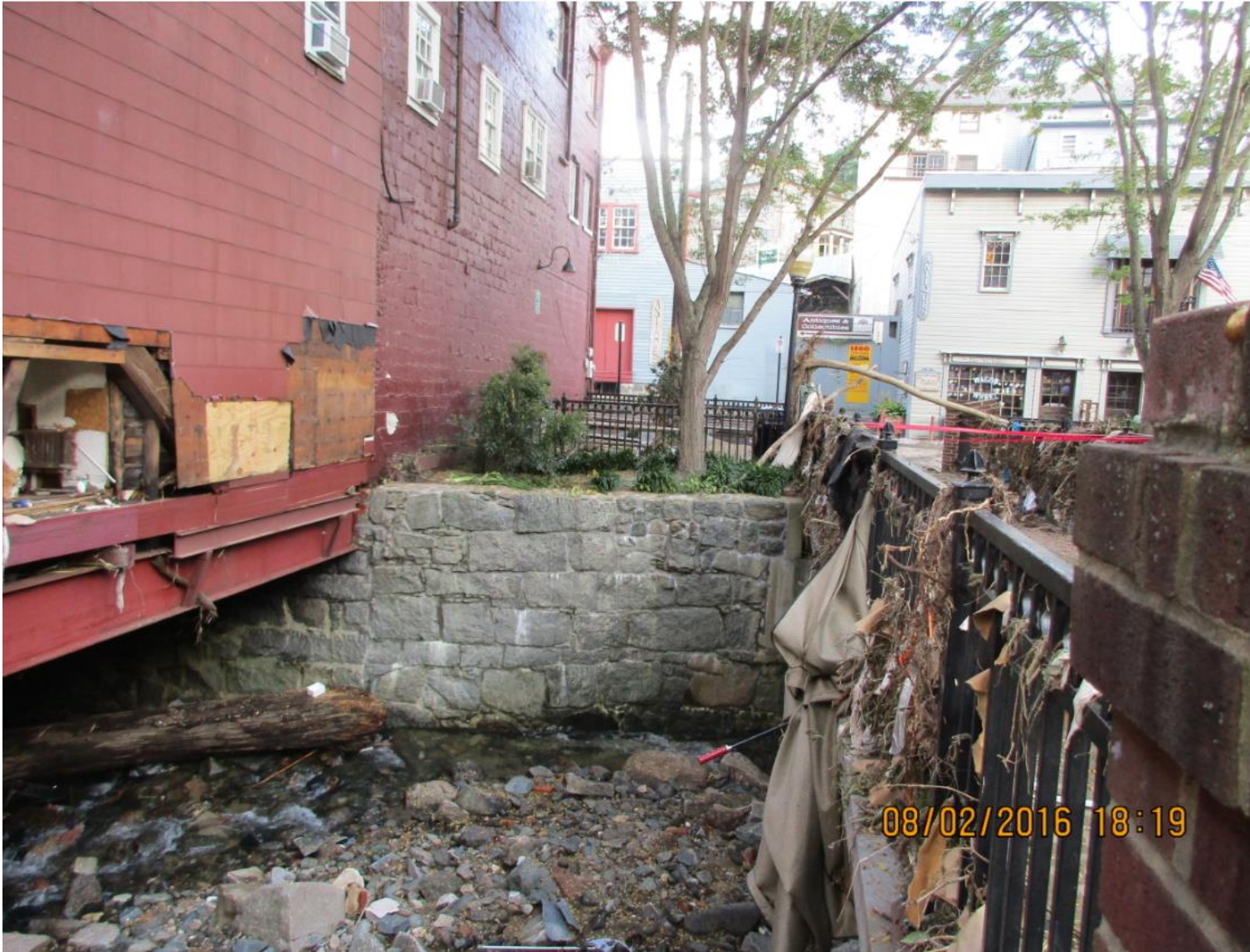
8059 Main Street west side of building and Tiber Park east side of bridge - Post 2016 flood
