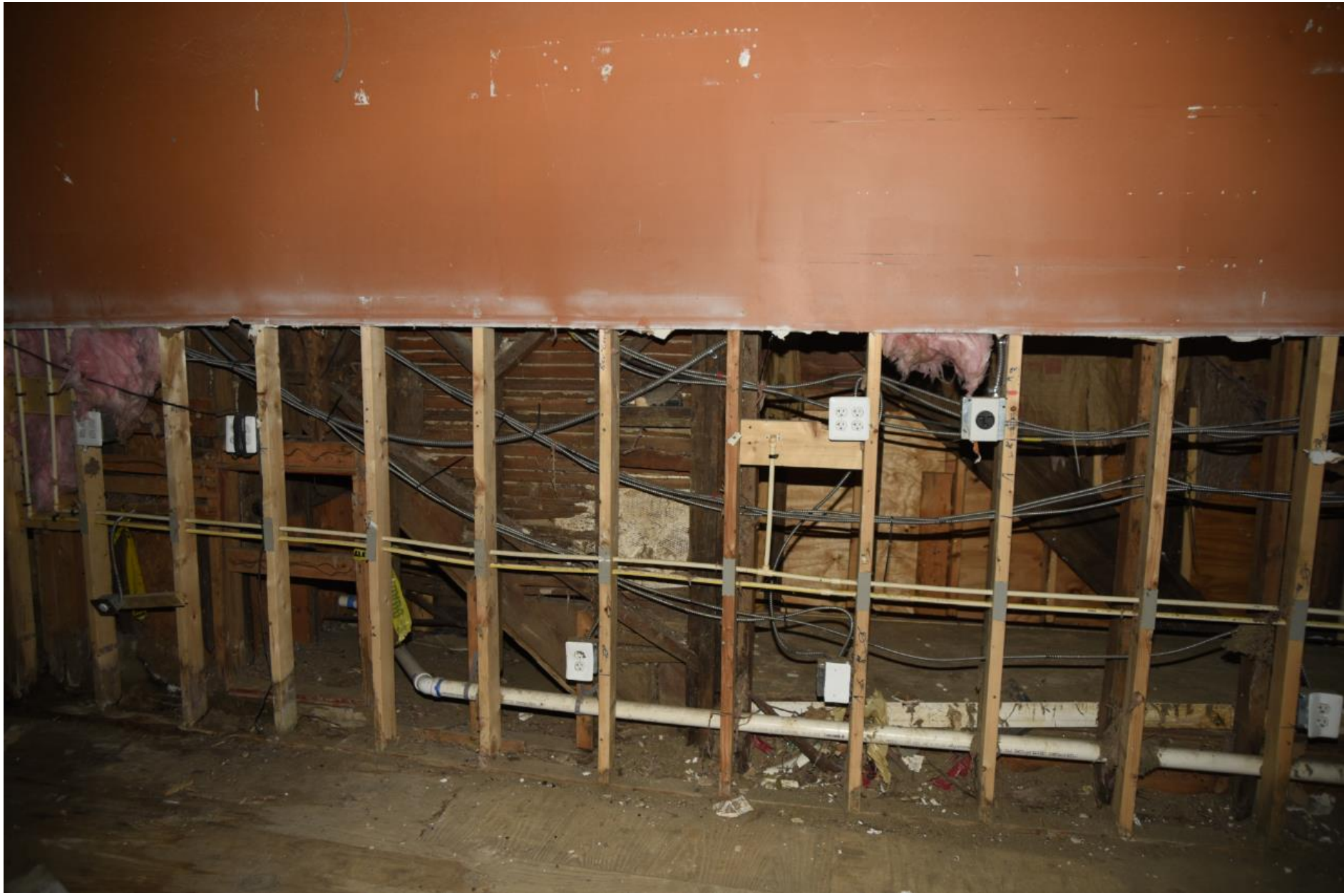
8059 Main Street interior damage.
