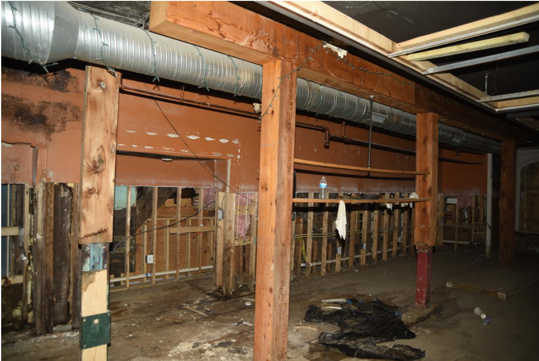
8059 Main Street interior damage.
