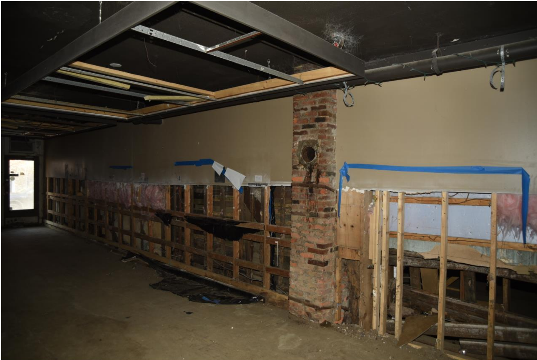
8059 Main Street interior damage.
