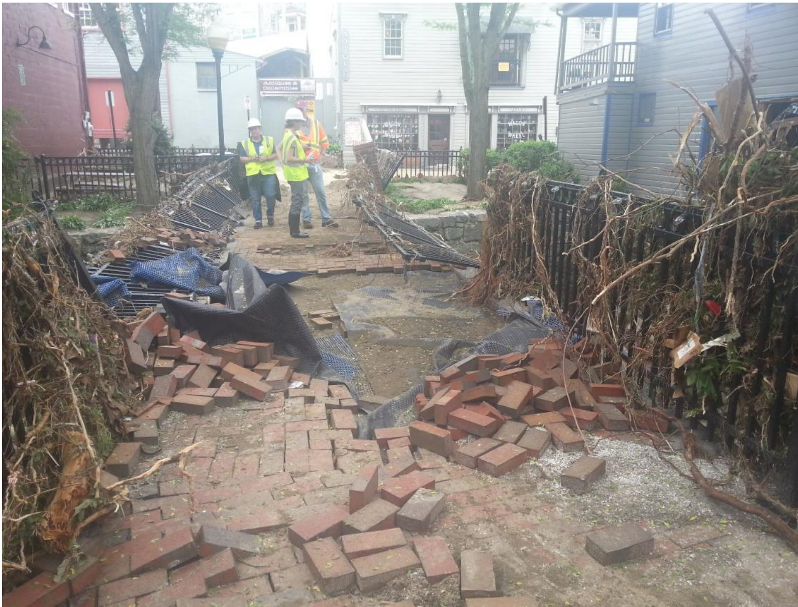
View of Tiber Park Bridge looking south toward Tiber Alley from Main Street – Post 2018 Flood
