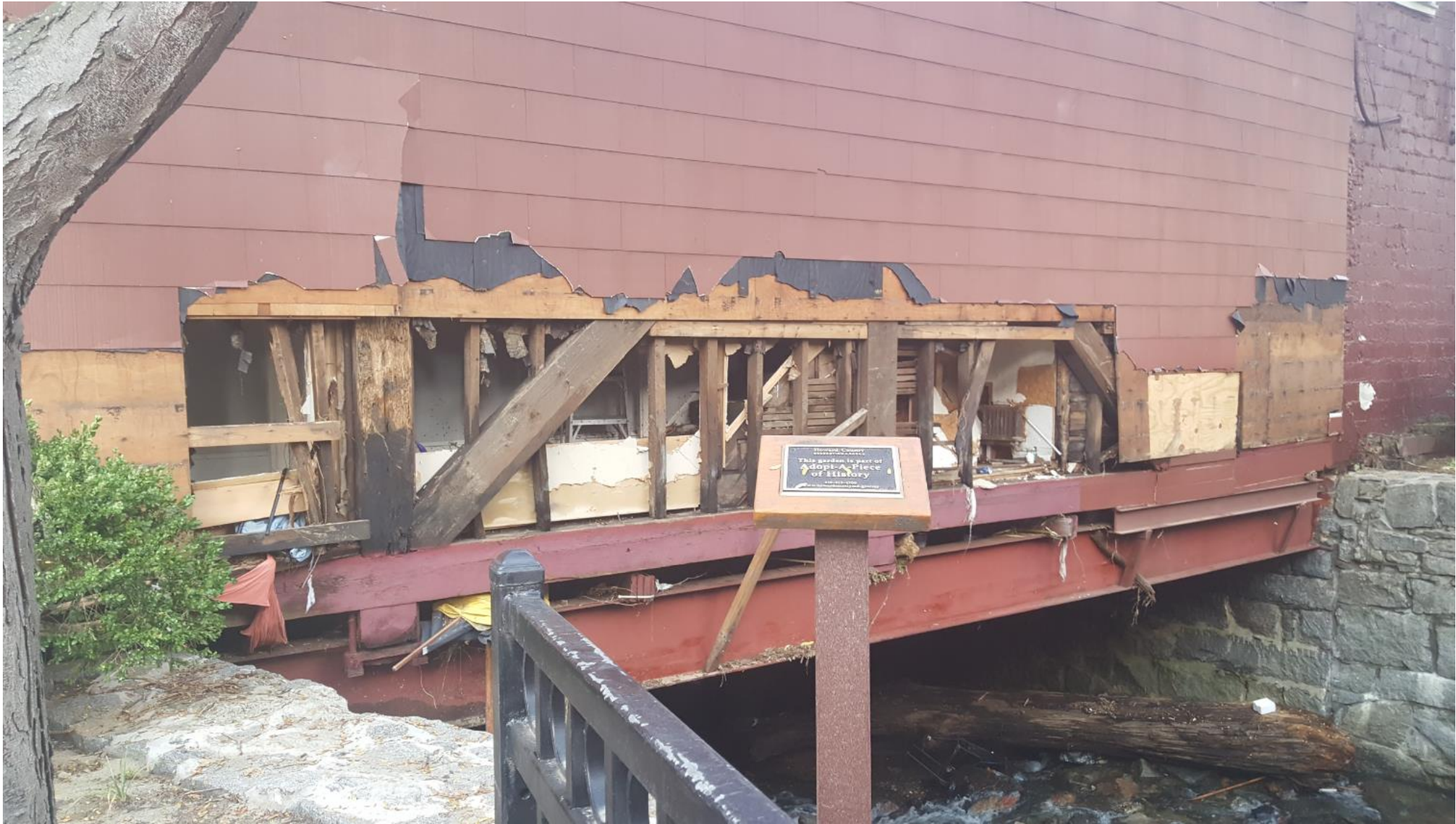
8059 Main Street west side of building - Post 2016 flood
