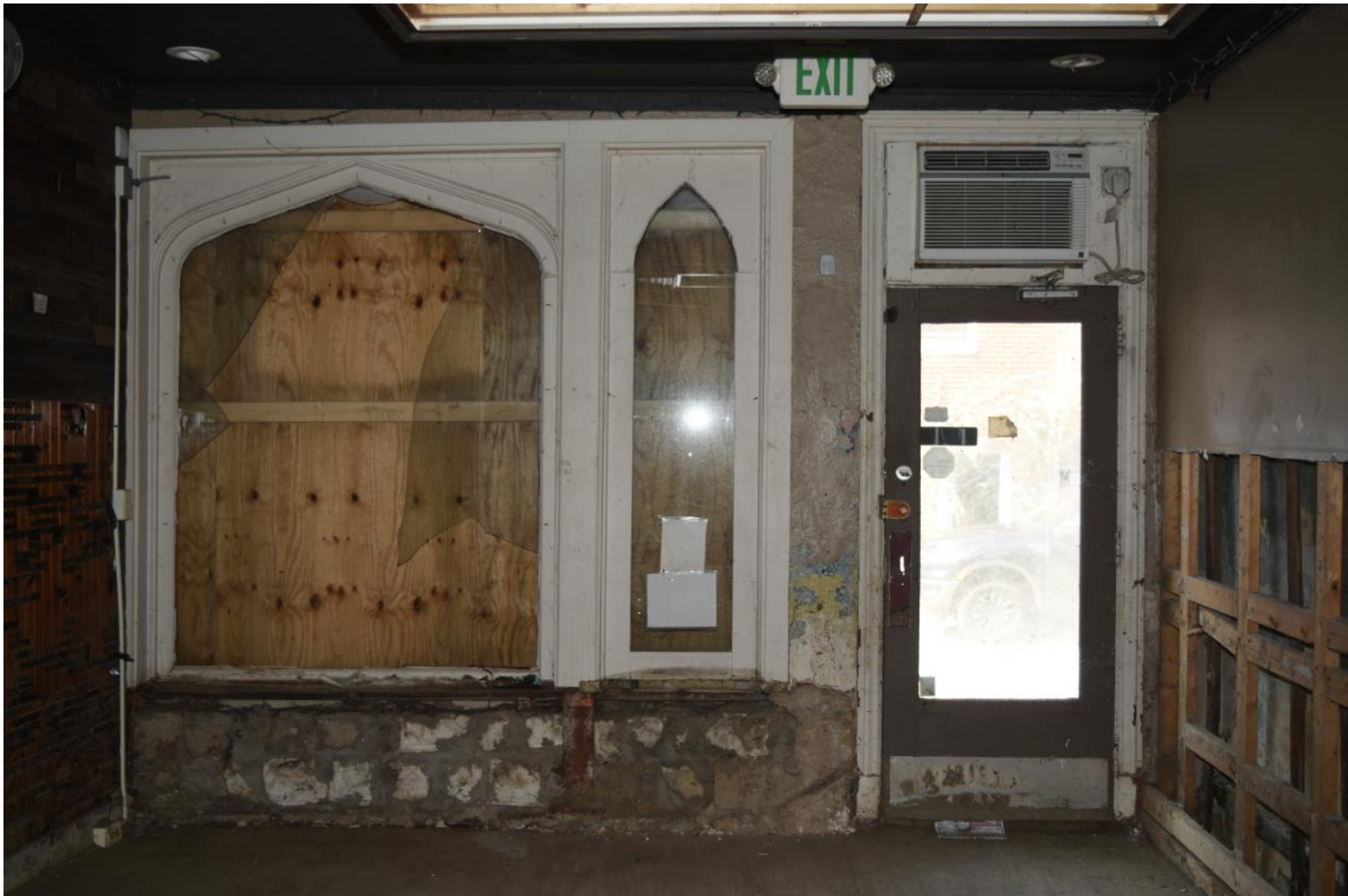
8059 Main Street interior damage.
