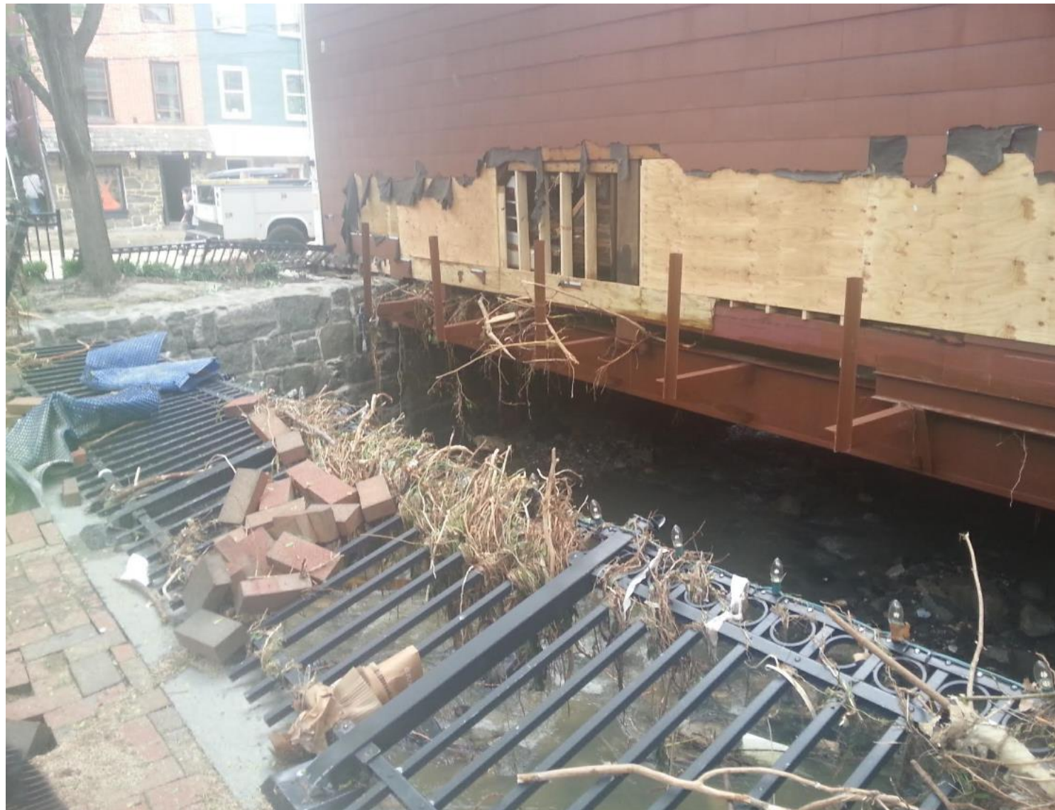
8059 Main Street west side of building - Post 2018 flood
