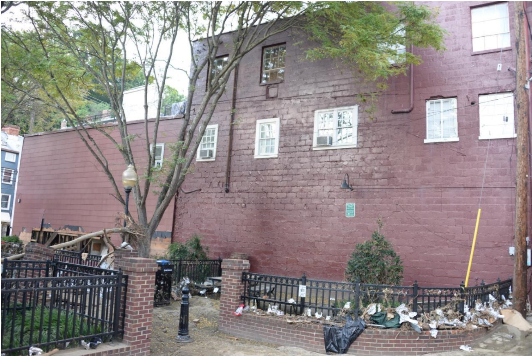
View of Tiber Park Bridge/west side of 8059 Main Street as seen from Tiber Alley looking north toward Main Street – Post 2016 Flood
