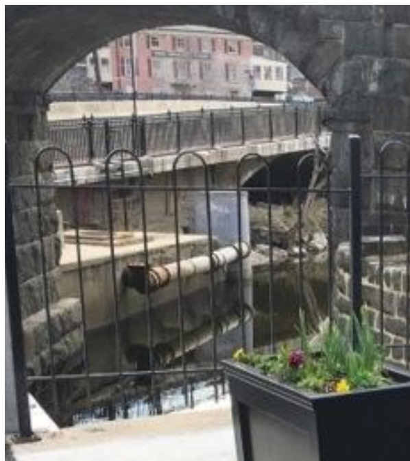
Figure 134: The Oliver Viaduct’s Narrow Opening Restricts Flood Conveyance in Lower Main
