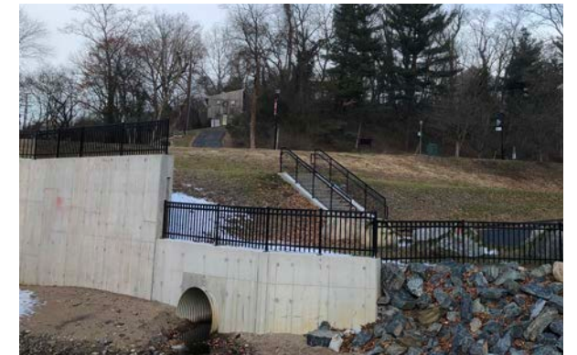
Figure 46: Existing Culverted Stream Outfall in Lot F After the Reconstruction Following the 2018 Flood
