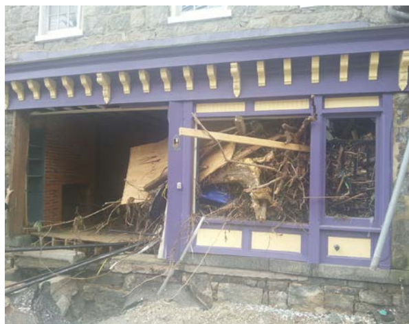
Figure 38: Vulnerable Tree Cover Along Stream Edges Creates the Potential for Debris Mobilization and Damage Downstream (Top); Tree Lodged in Building (Bottom)
