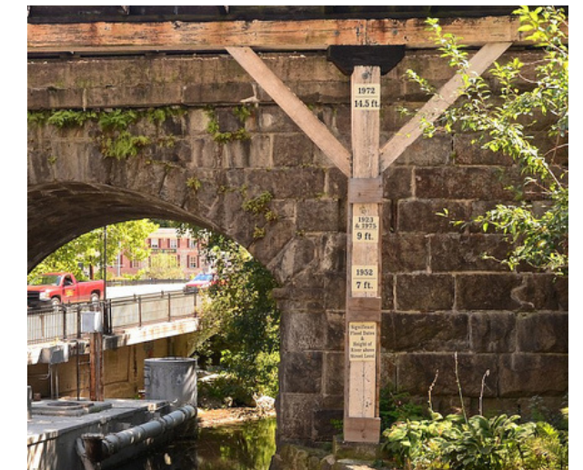
Figure 43: High Water Mark in Ellicott City on the Oliver Viaduct (Pre 2016 Flood), Credit Frank Monaldo
