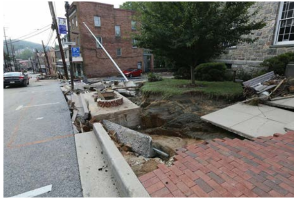
Figure 95: Damage to Brick Paving after the 2018 Flood
